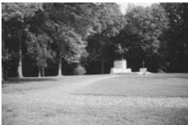
FIGURE 65. Grass growing up between the brick joints on the amphitheater's northern radial walk.
