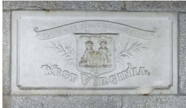
Figure 14. Rusted iron wedges in top and bottom joints, West Virginia. [2000 image.]
