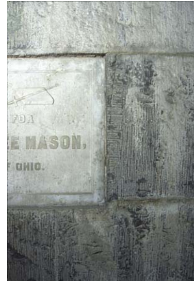
Figure 12. Remains of flashing in joint above Masons, Grand Lodge of Ohio. Note absence of thick calcite crust on stone, to right side of stone, and beneath stone. [2000 image.]
