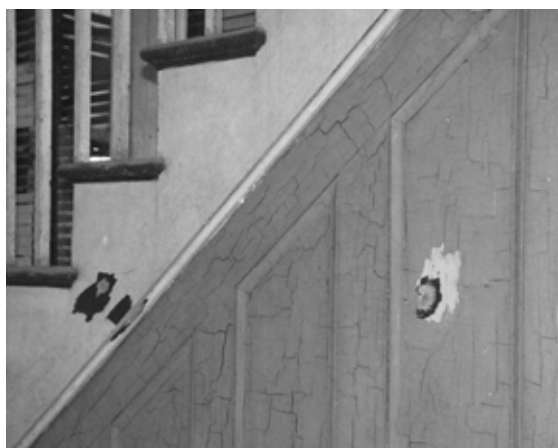
Figure 46 View of original woodwork on staircase, with scraped areas exposing the brown paint used in 1902. NPS SERO 2001.
