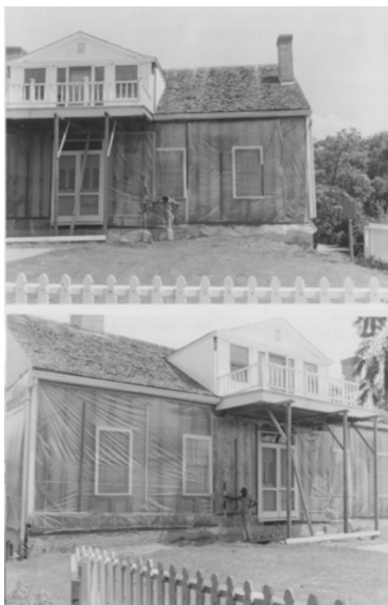
Figure 29 Views of front of house after removal of exterior siding to investigate structural condition, July 1965. VICK Coll.
