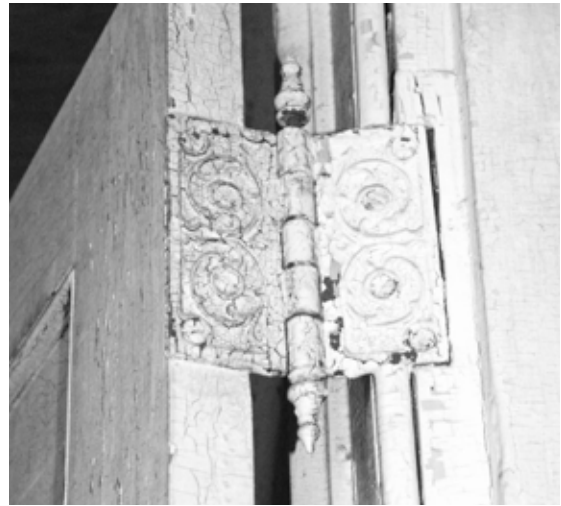
Figure 48 View of "fancy" hinges originally used at most primary doors. NPS SERO 2001.
