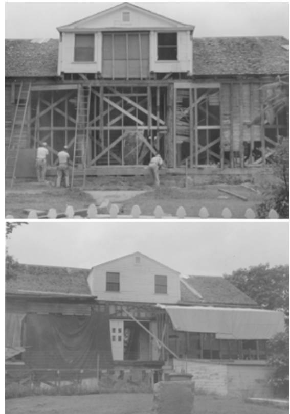
Figure 30 Views of front (upper image) and rear (lower image) of house, May 1966. VICK Coll.
