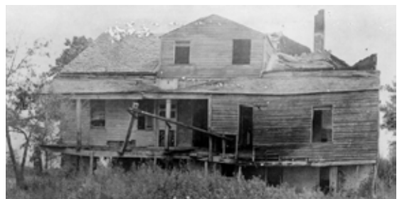
Figure 8 View of rear of house, 1900. Note collapsed roof on west side. HABS File No. MISS, 75-VICK. V. 3-7.
