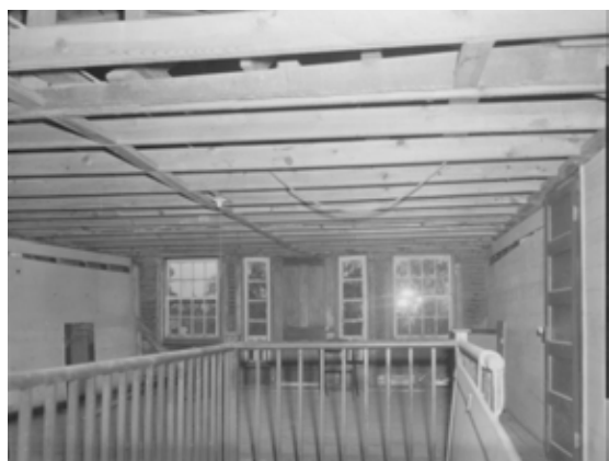
Figure 25 View north in Room 200 after removal of fiber-board ceiling, November 1965. VICK Coll.
