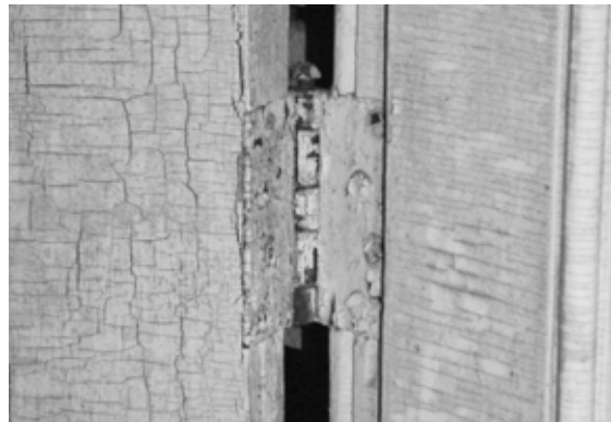
Figure 49 View of butt hinges used at folding doors. NPS SERO 2001.
