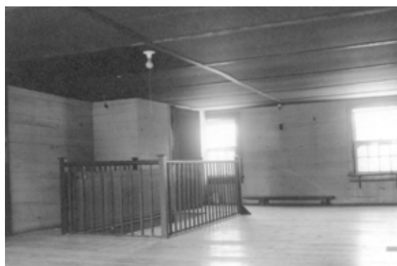
Figure 18 View north in Room 200, May 1965, showing fiber board ceiling installed by Major Holt in 1931. VICK Coll.
