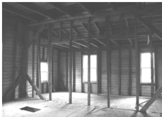
Figure 57 View northwest in Room 102, looking through wall framing into Room 103. NPS SERO 2001.
