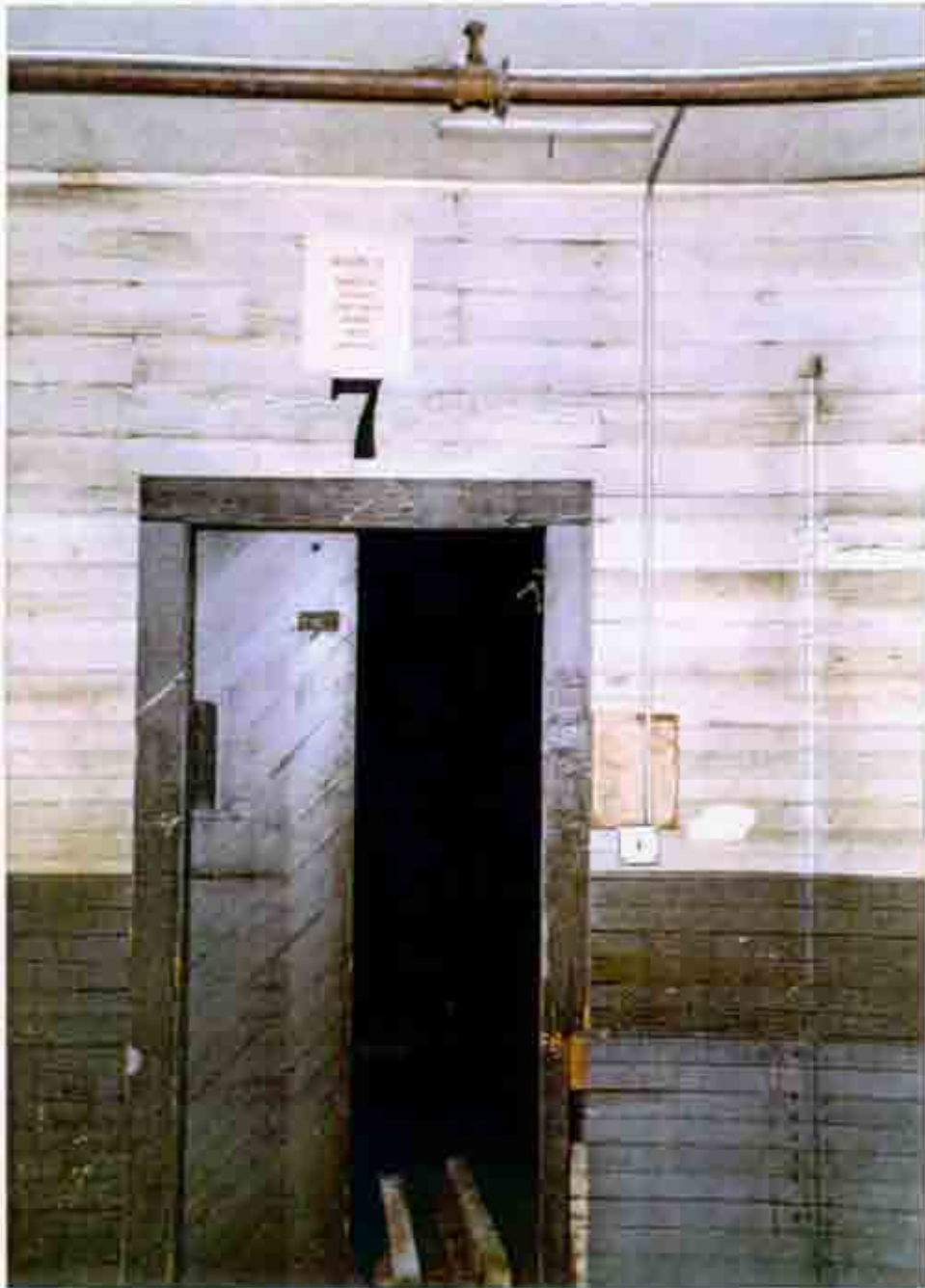
Figure 3.15 Detail of the wood partition and typical door, installed by the Williams Baking Company.
