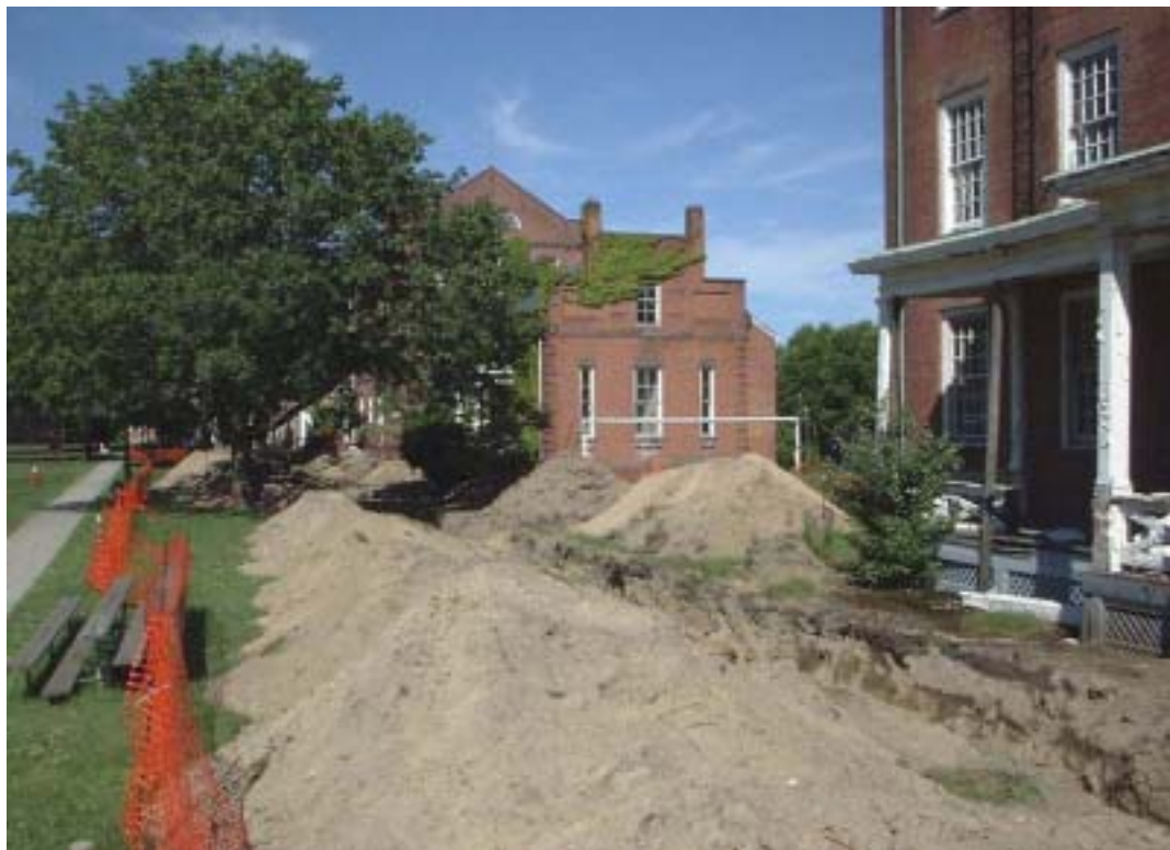
Figure 38. Trench along length of the south side of the Green, 2002 (OCLP SPAR CLI File).
