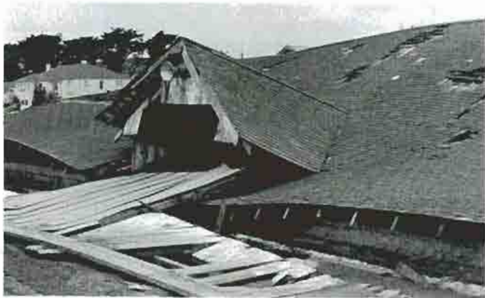
Nunes Ranch hay barn after a storm, 1982. The demolished structure was removed by the Nunes'. Courtesy of the Point Reyes Light .
