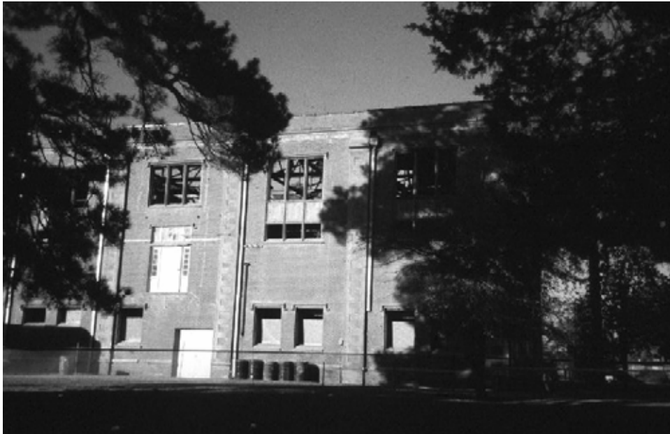
Figure 51. North façade (top) and south façade (bottom) of NCPTT's Nelson Hall (former Women's Gymnasium after the fire, 1997 (NCPTT)).
