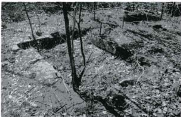
FIG. 12. FOUNDATION OF A WORKER'S HOUSE, DOLPH/SUNNYSIDE INDUSTRIAL DISTRICT. PHOTOGRAPH COURTESY OF CHRIS, INC., NORTH WALES, PA.
