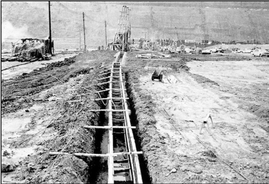
Figure 8-8: Seepage into the earthfill section of Kinzua Dam was prevented by constructing a trench three feet wide, 1100 feet long, and up to 160 feet deep on the upstream side. This was then filled with bentonite slurry to stabilize the side walls and then filled with concrete placed through pipes from the bottom up displacing the bentonite slurry. Source: Pittsburg District, U.S. Army Corps of Engineers.
