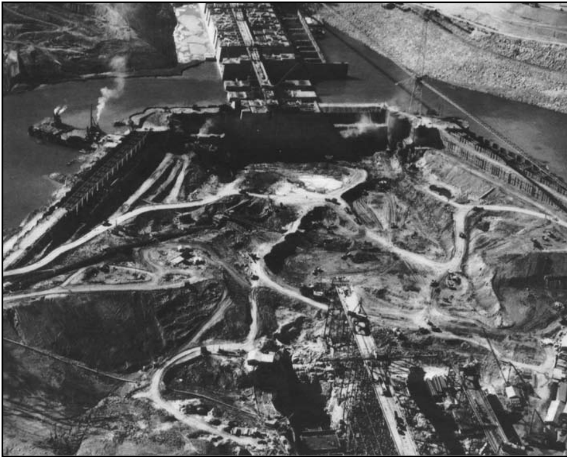
Figure 5-23: Excavating to bedrock behind the west cofferdam at Grand Coulee in 1936. Source: Bureau of Reclamation.
