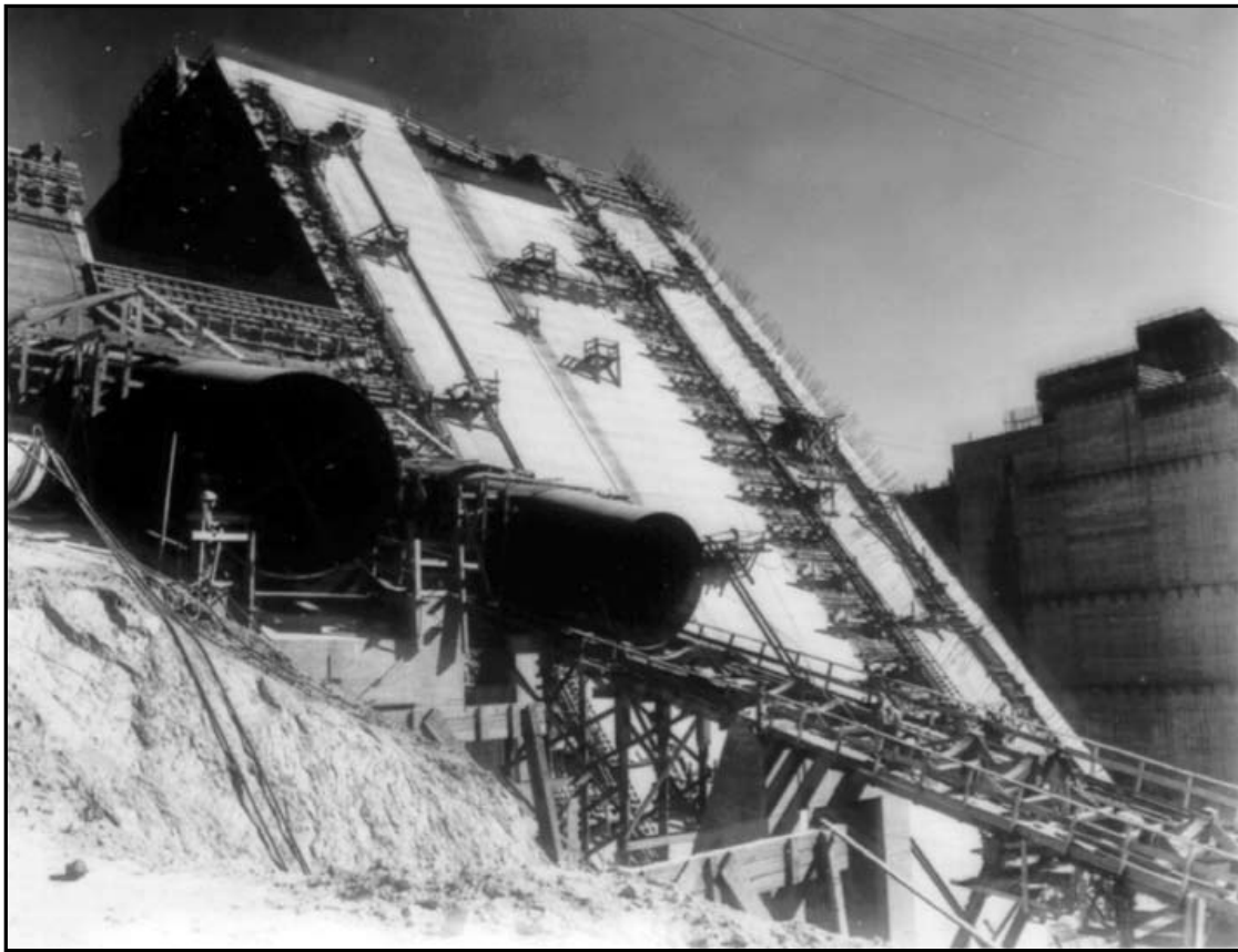
Figure 7-7: This 1942 construction photo shows the right abutment on the downstream face of Shasta Dam, during the placement of penstocks. Source: Bureau of Reclamation.
