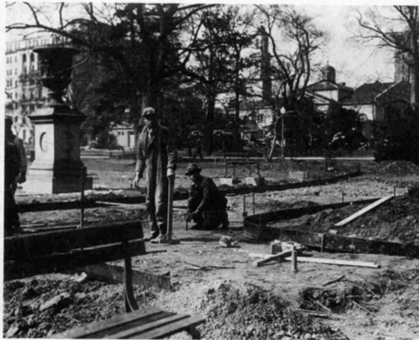
Fig. 32.--View looking toward St. John's Church (the "Church of the Presidents") and Sixteenth Street, showing relocated urn and workmen enlarging walks at east or Madison Place entrance to Lafayette Park, March 1936.
