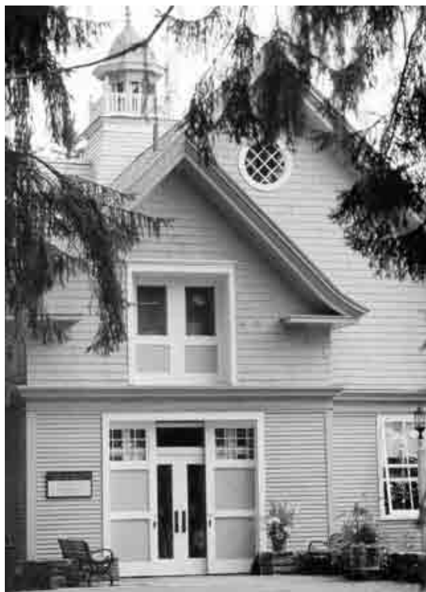
Figure 7.3: View of the front of the Carriage Barn following rehabilitation into a visitor center and park offices. Marsh-Billings-Rockefeller National Historical Park, 1999. In the foreground is the new stone-paved entranceway.
