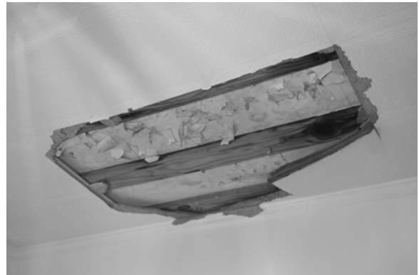
Figure C-27 Damaged modern ceiling tile
