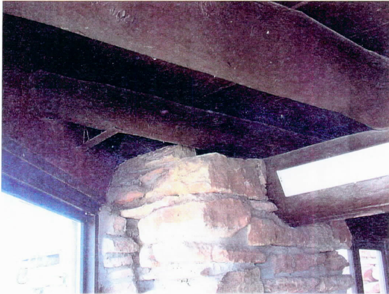
CRITICAL CONNECTION FROM INTERIOR
