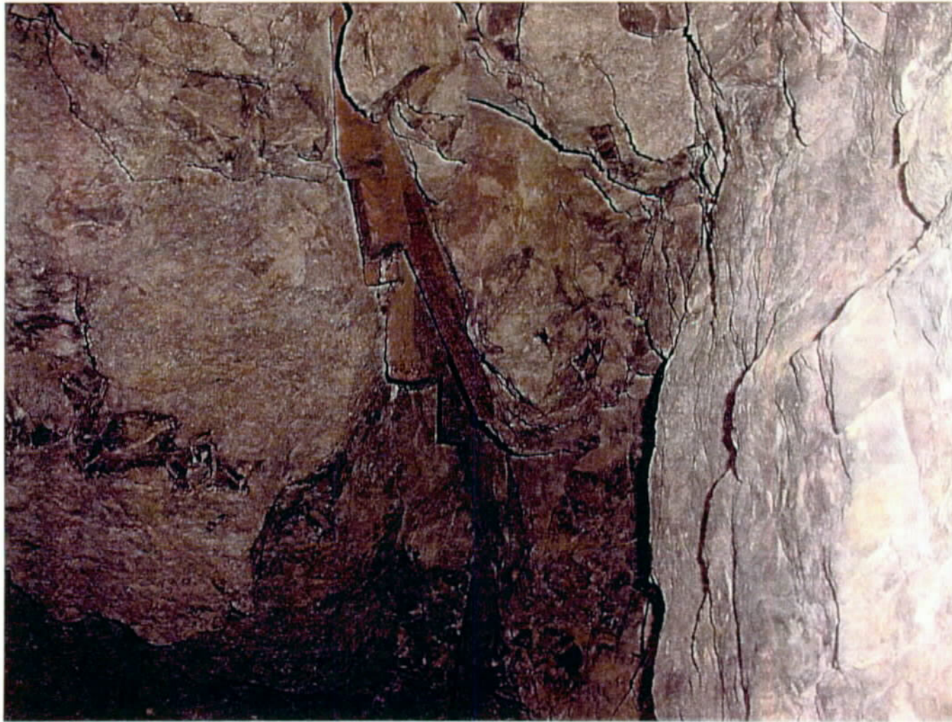
BASEMENT, SHOWING CONTINUING CRACK AND WOODEN WEDGES
