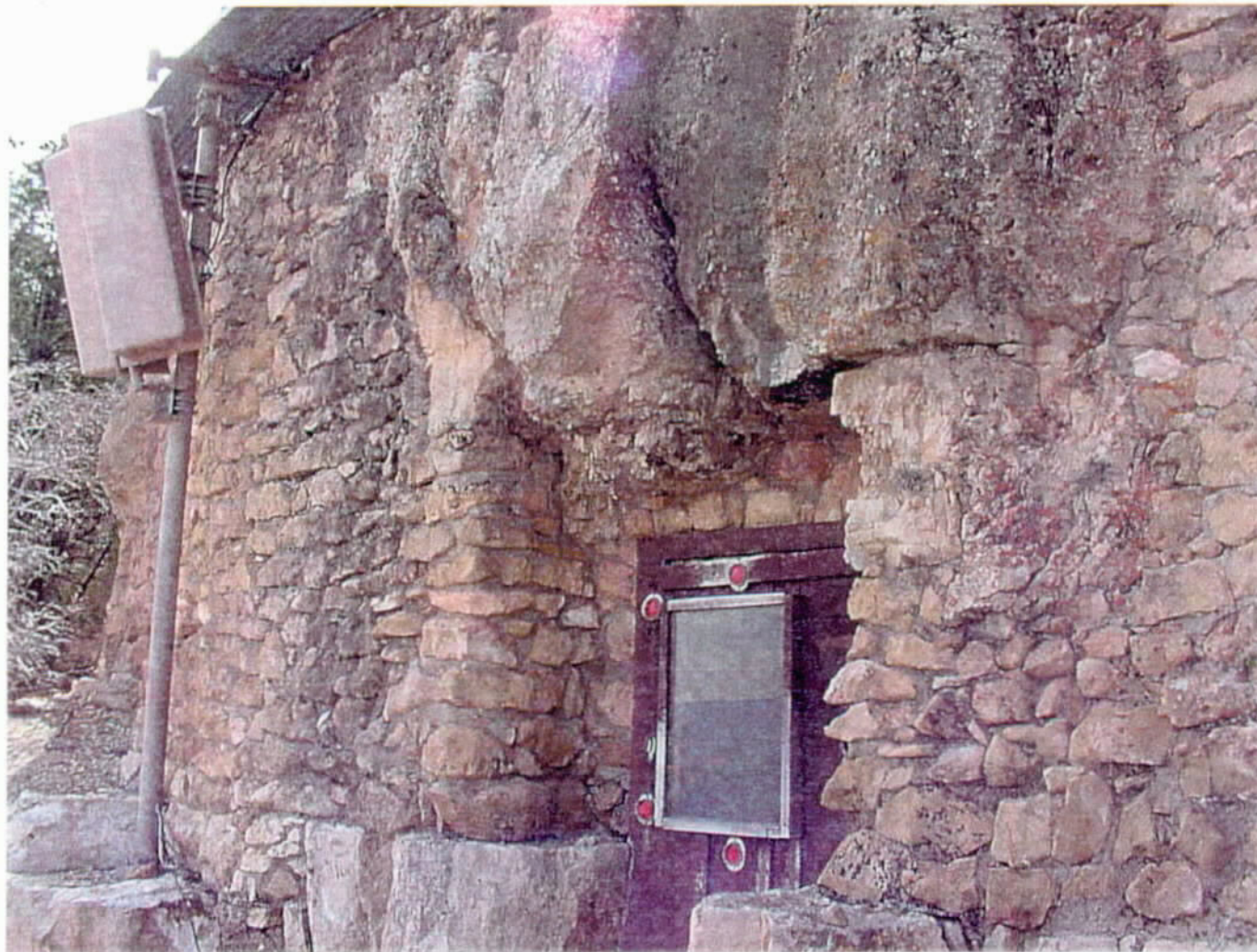
BASEMENT, SHOWING CRACK AND MASONRY REPAIRS TO CANYON WALL
