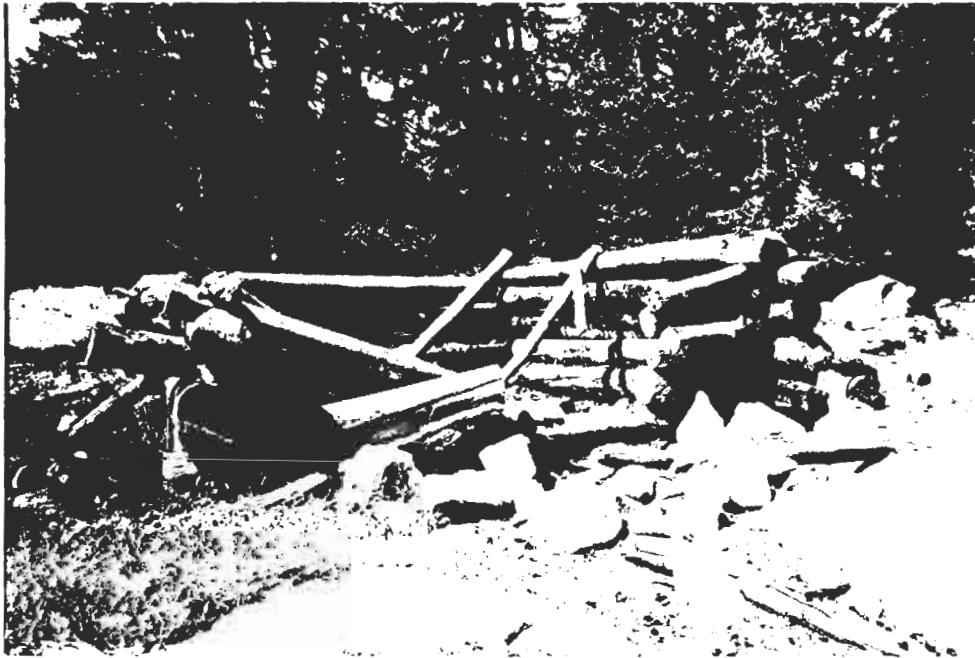
Partially Collapsed Log Building at Johnson Mine Just Below Johnson Lake
