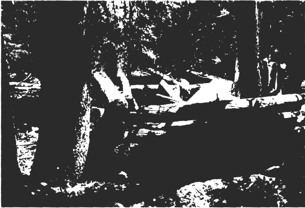
Partially Collapsed Two-Room Log Cabin at Johnson Mine Just Below Johnson Lake
