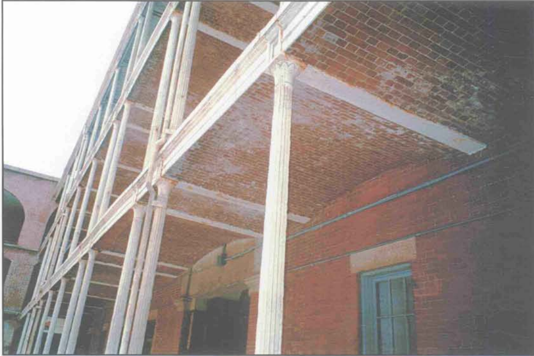
Condition Photo 10: Southeast Face Courtyard; Corroding metal columns and walkway supports. Missing metal railings in this photo have been reinstalled. (Courtesy of ARG, 2003)
