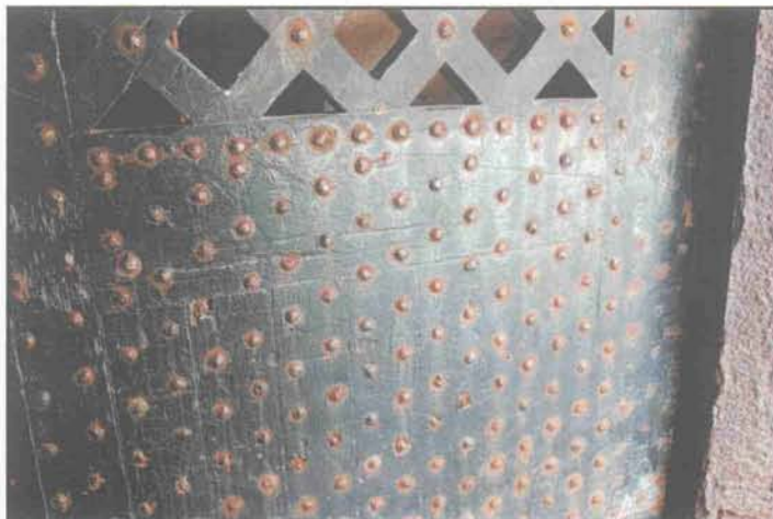
The rivets on the original wood doors rust quickly in the marine environment. (John Martini, 2005)
