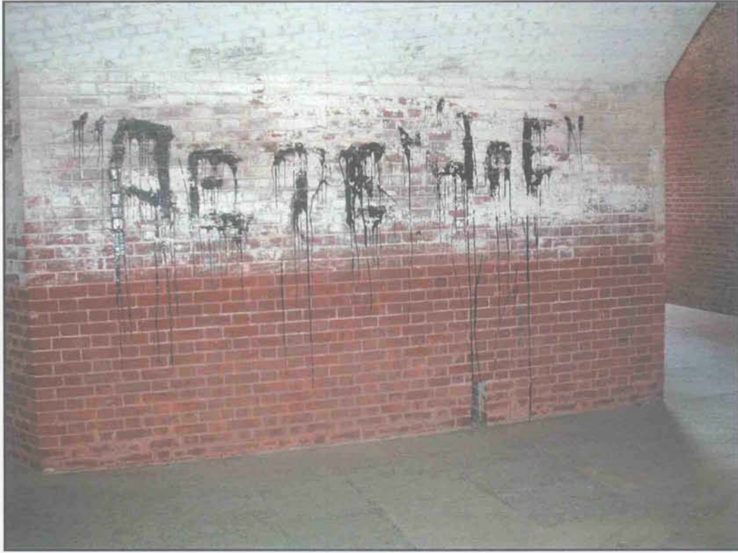
Condition Photo 18: Casemate 68A—Second Tier; Graffiti noted on masonry wall. (Courtesy of ARG, 2003)
