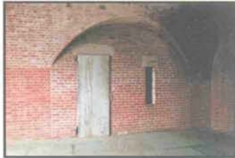
This wall was added to convert three 3rd tier casemates into a jail cell. (John Martini, 2005)
