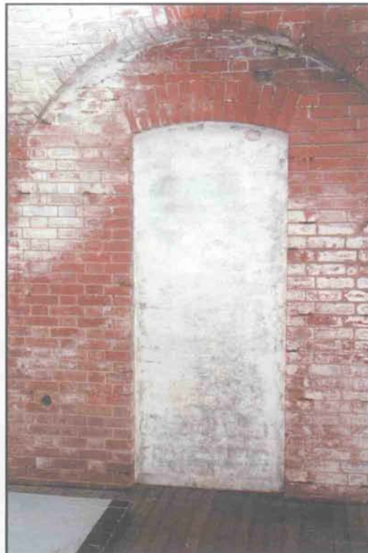
The original doors and brick infill walls are visible in the 3rd tier stores. (John Martini, 2005)
