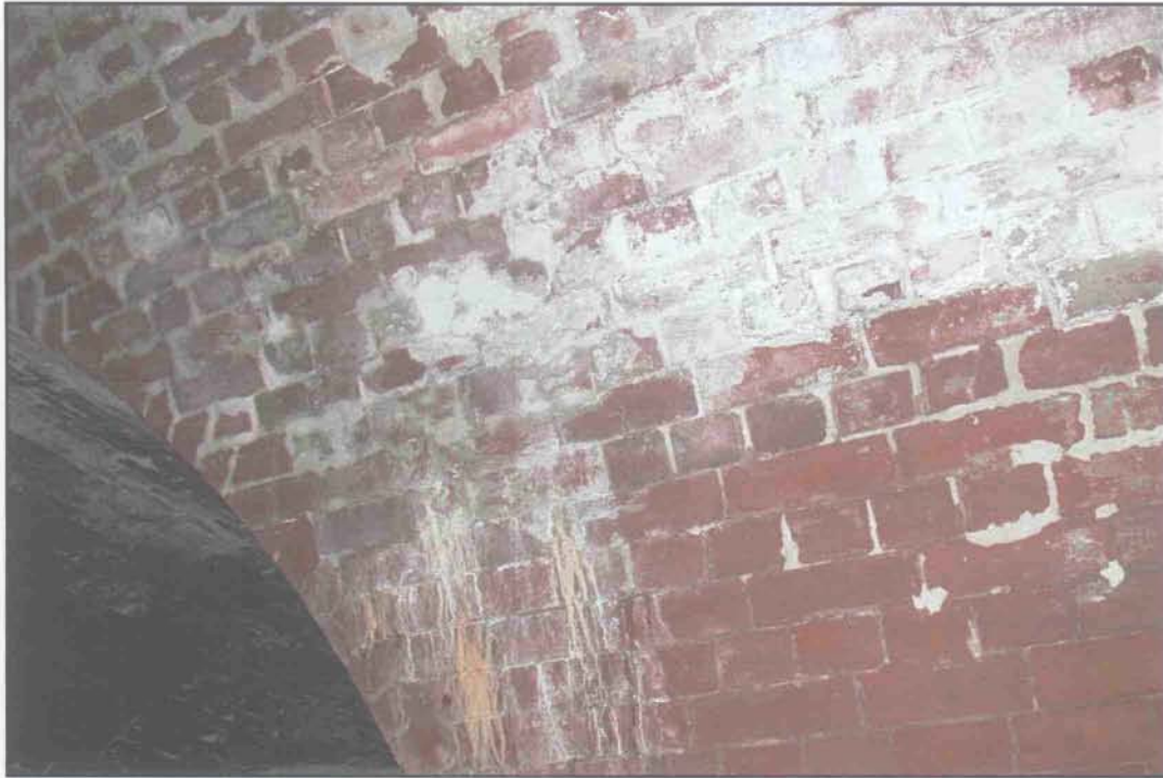
Condition Photo 3: Casemate 101; Calcium deposits are draining from open joints and coasting is no longer extant. (Courtesy of ARG, 2003)
