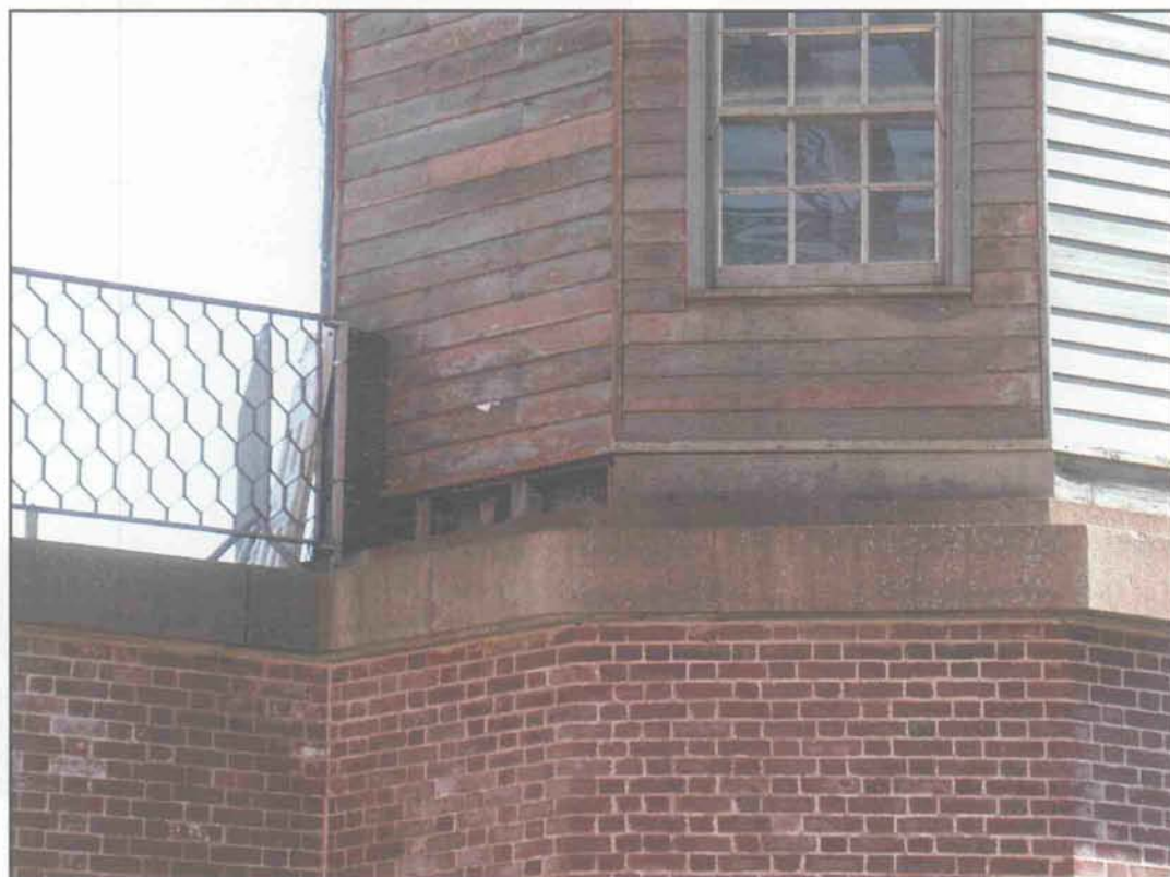
Condition Photo 13: Stair 3; Missing siding exposes the structural framing. (Courtesy of ARG, 2003)
