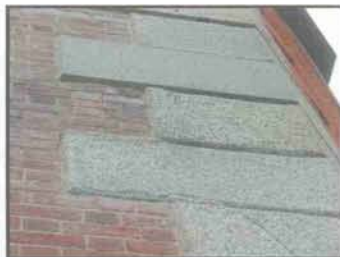
The quoins in the path of the wind and saltwater spray have lost their smooth quarried finish. (Jane Lehman, 2005)
