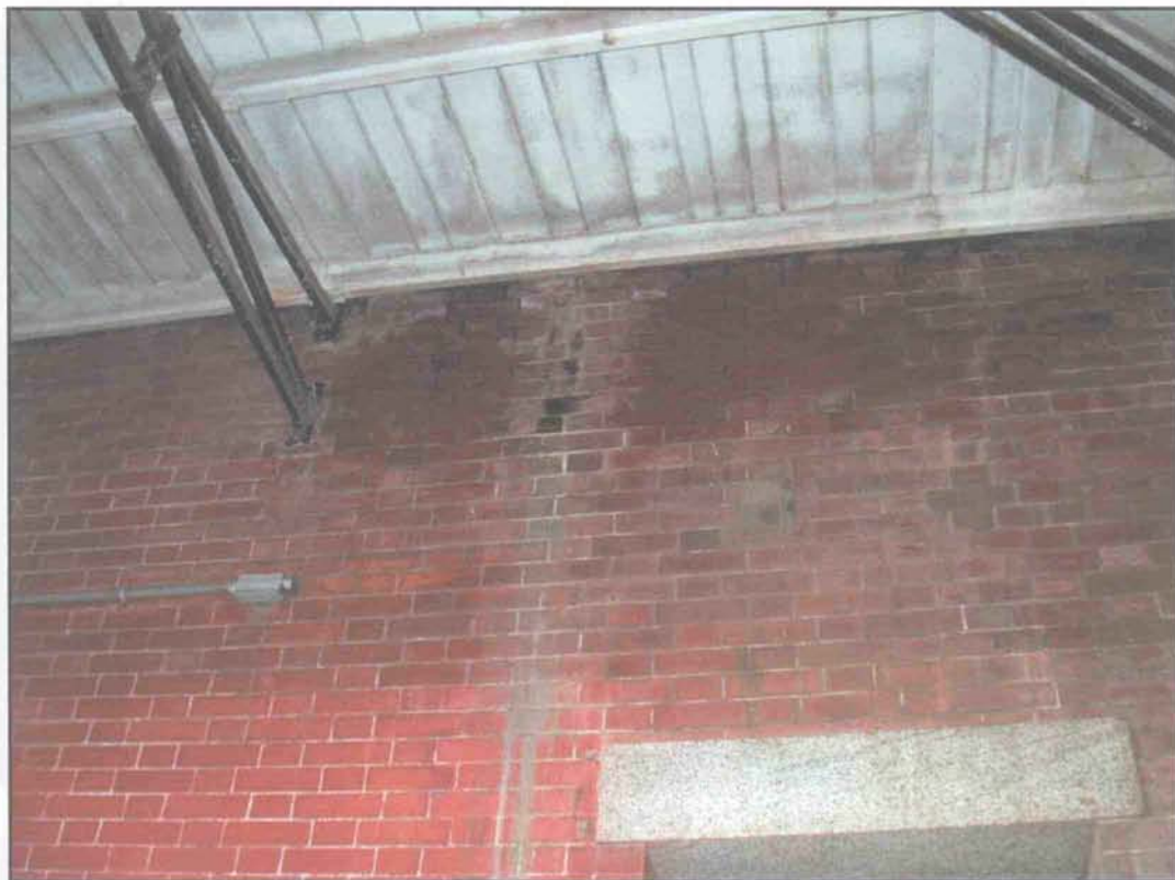
Condition Photo 12: Southwest Courtyard Elevation— Third Tier by Stair 1; Roofing materials are saturated from improper drainage at the barbette tier. The wood appears to be deteriorated. Biological growth has settled on the roofing materials and the masonry. Paint coatings are no longer extant. (Courtesy of ARG, 2003)
