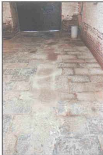
The original granite floors remain in good condition although a large concrete patch exists where a previous water line was installed. (John Martini, 2005)
