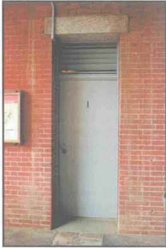
The transom windows above the 3rd tier gallery doors were replaced with wood louvers. These louvers need to be replaced because they are all installed backwards. (John Martini, 2005)
