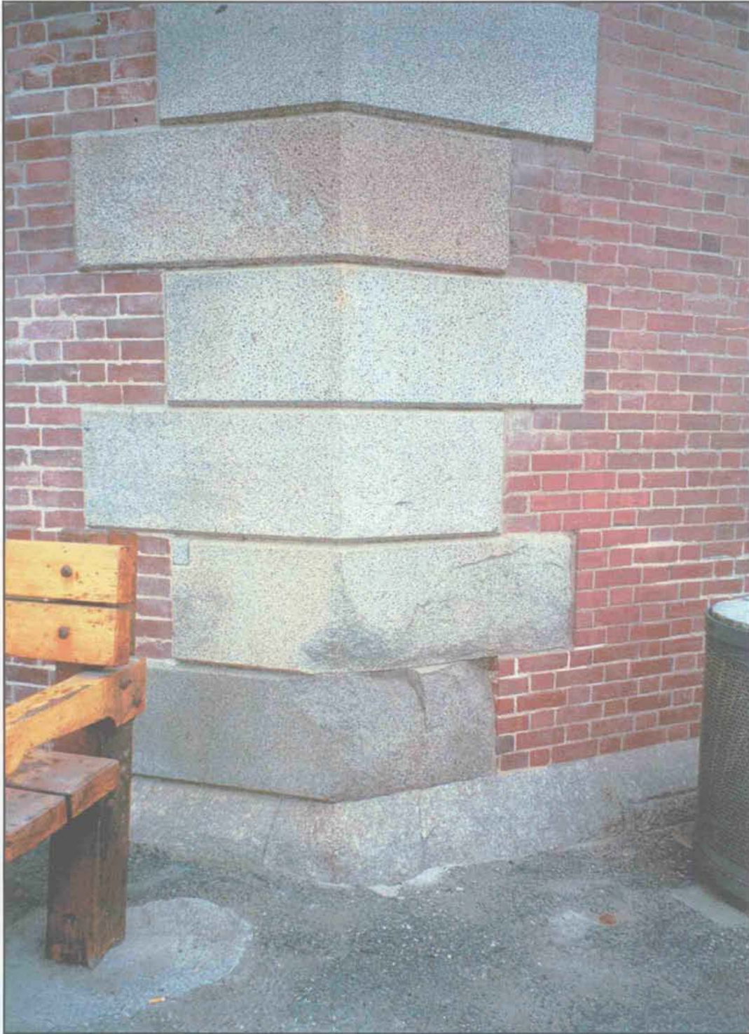
Condition Photo 7: East Bastion—East Flank; Impact damage at granite quoins and base. (Courtesy of ARG, 2003)
