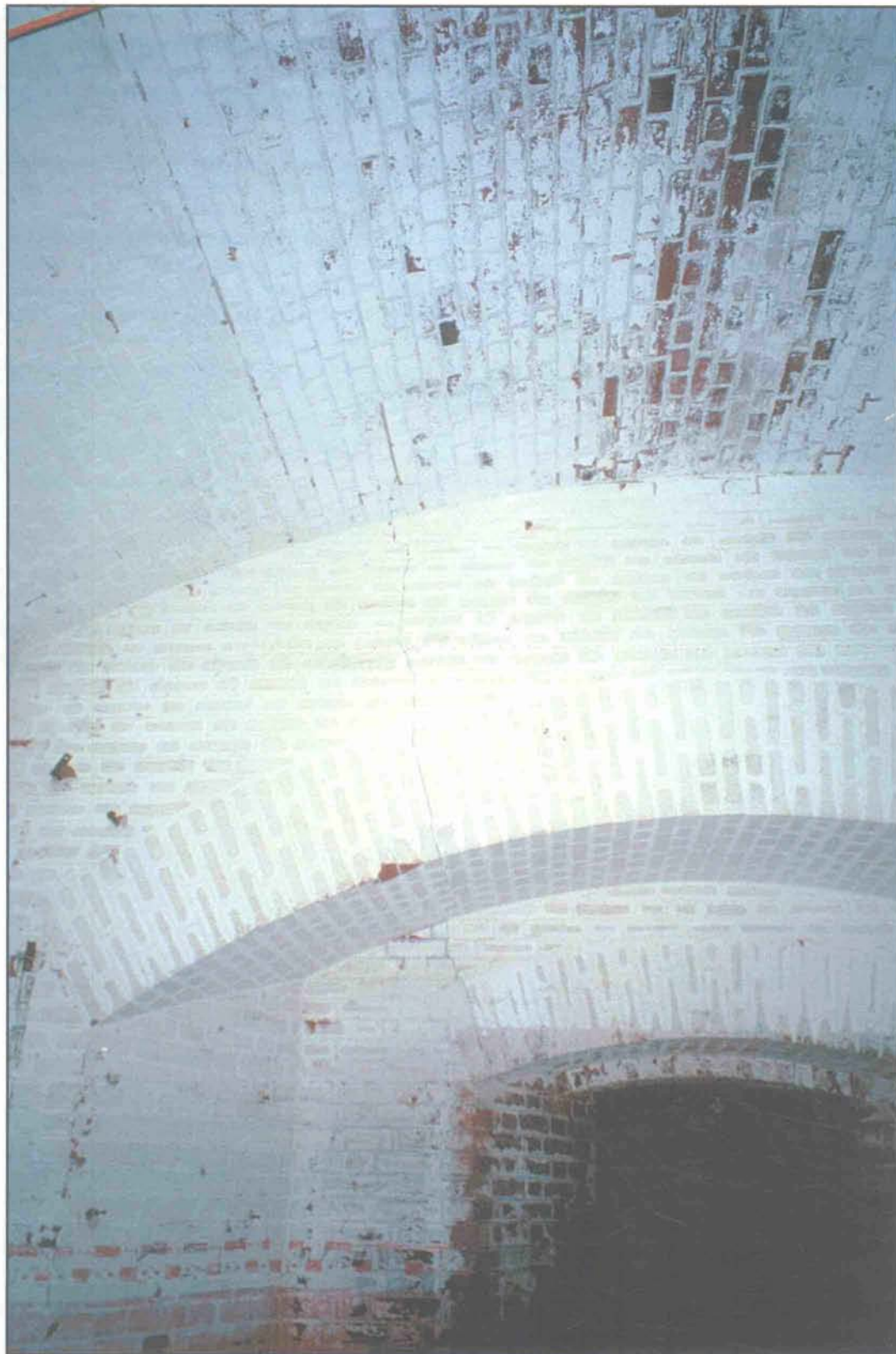
Condition Photo 15: Casemate 19; Cracks in brick masonry and joints have failed. The heavily flaking paint is typical in casements. (Courtesy of ARG, 2003)
