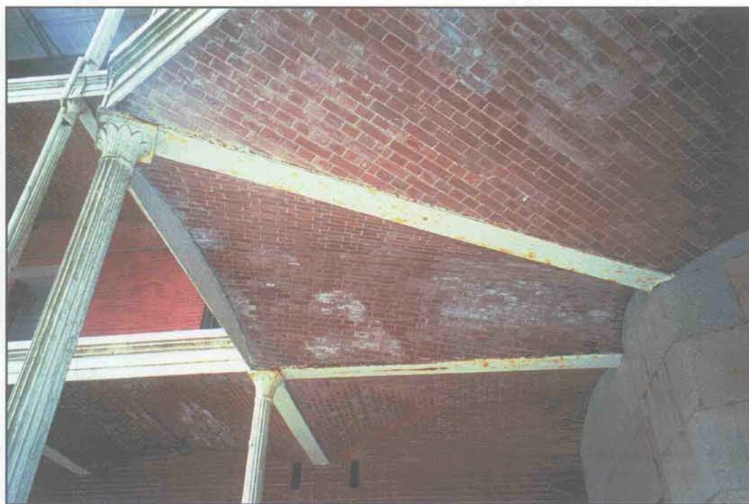
Condition Photo 9: Southeast Courtyard—Underside of Walkway at Tier One; Metal corrosion and staining of the granite walls. The brick facing is spalling. Efflorescence occurs on the brick and granite masonry. (Courtesy of ARG, 2003)
