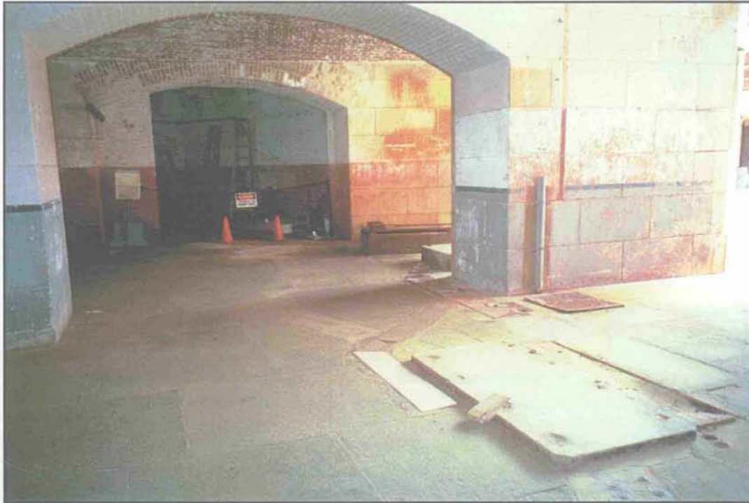
Condiiton Photo 19: Casemate 34; Uneven surfaces, open holes and potential tripping hazards. (Courtesy of ARG, 2003)
