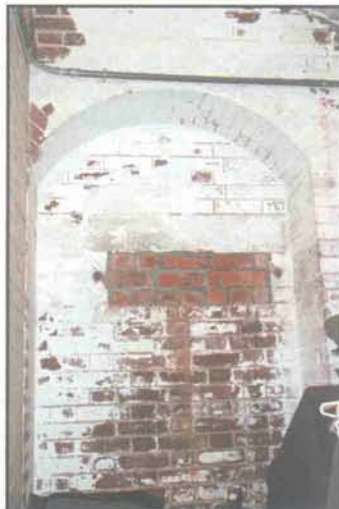
The rifle slit in the corridor of the jail area has been infilled with brick. (John Martini, 2005)
