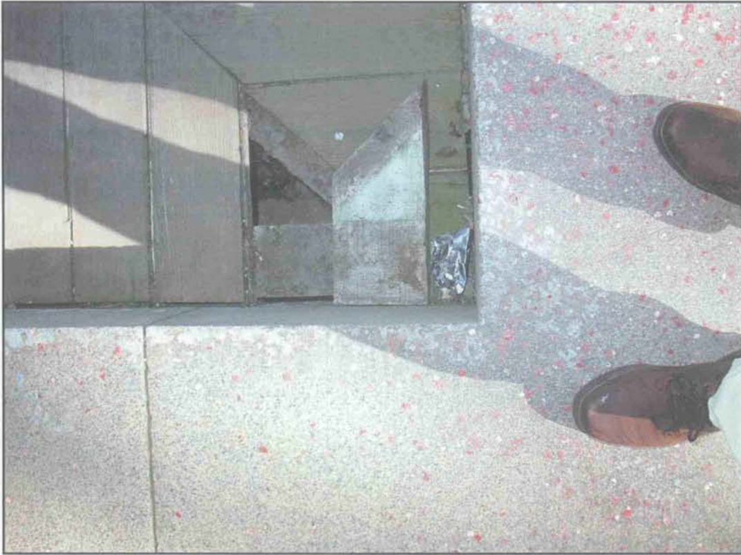
Condition Photo 14: Wood Walkway – Barbette Tier by Stair 1; Components are not properly fastened at wood walkway. (Courtesy of ARG, 2003)
