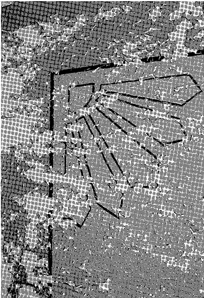
Figure A-20. Ceiling stencil (corner detail), Stairway #5, southeast corner of lobby, second floor. (Photograph by J. Quinn, March 1994.)
