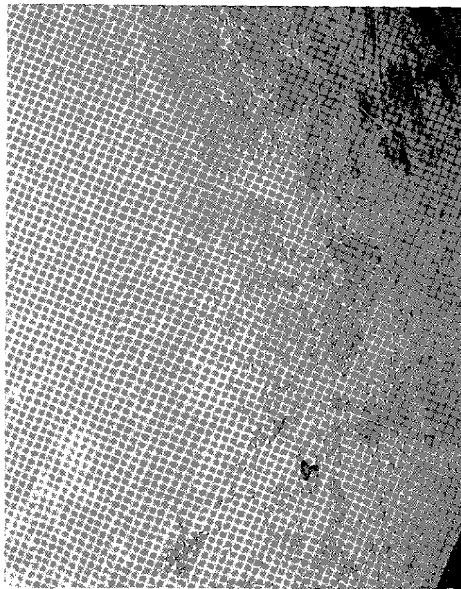
Figure 190. Imitation Caen stone stucco finish along north wall of Stairway #2; scoring of blocks visible.
