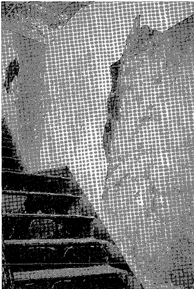
Figure 46. Imitation Caen stone on wall of Stairway #5 between second and third floors, showing pargeting spalling from scored cement brown coat.
