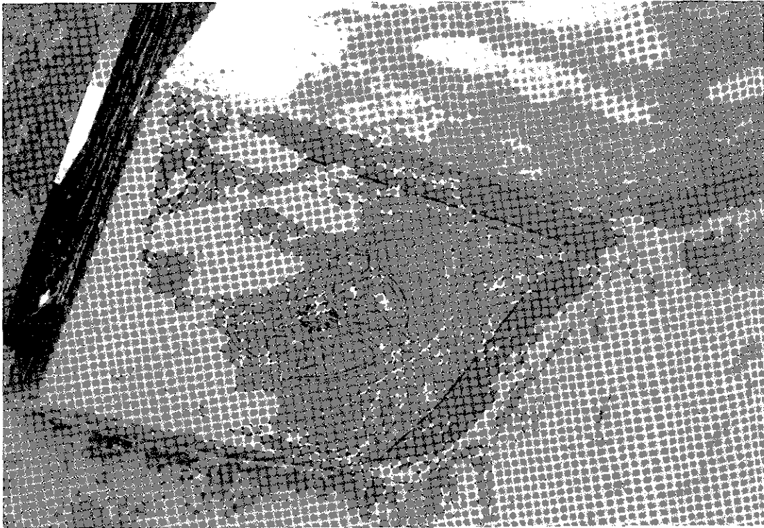
Figure A-18. Ceiling stencil, Stairway #3, northeast corner of lobby, second floor. (Photograph by Frank Matero, January 30, 1981.)
