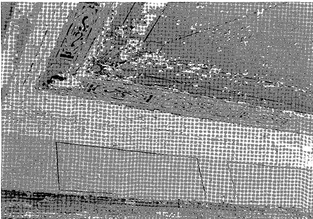
Figure A-15. Main ceiling stencil border and balcony frieze showing panels that once held painted canvases. (Photograph by Frank Matero, January 30, 1981)
