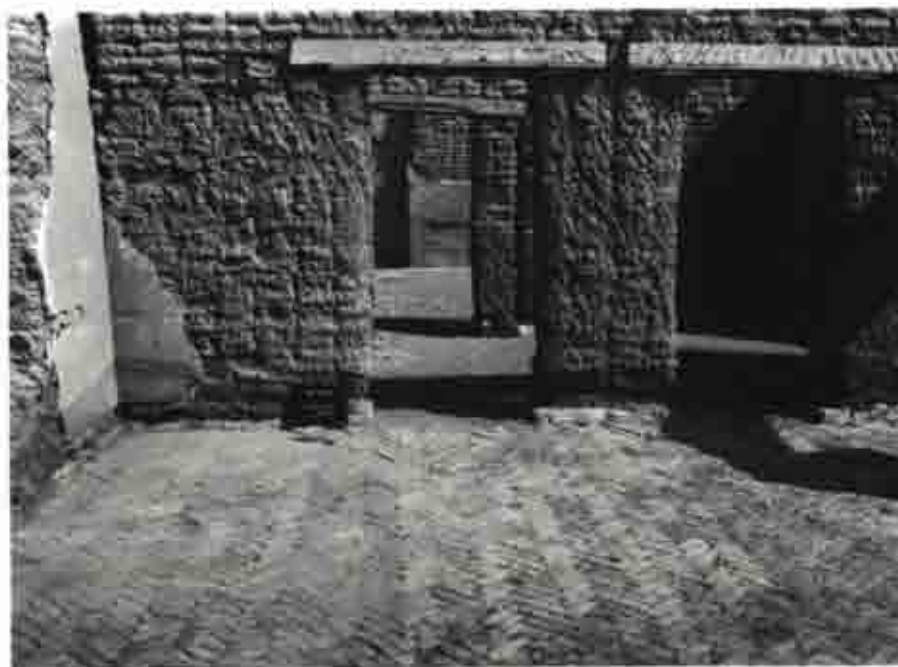
Figure 29. Photo, herringbone-pattern brick floor in Room 3-325 and east wall. [Cattanach 2/26/57, Neg FOUN-112(s)]
