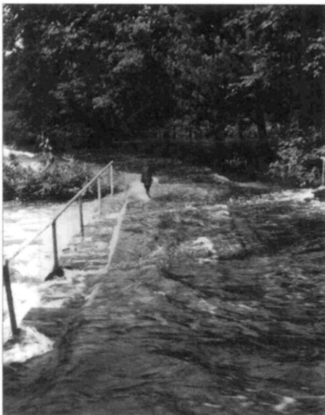
Figure 4.10. The bridge during a 1953 flood. Notice the pipe railings installed by Charles Curnan from supports from the old canvas awning of the pool terrace. FDRL 81 90 5.
