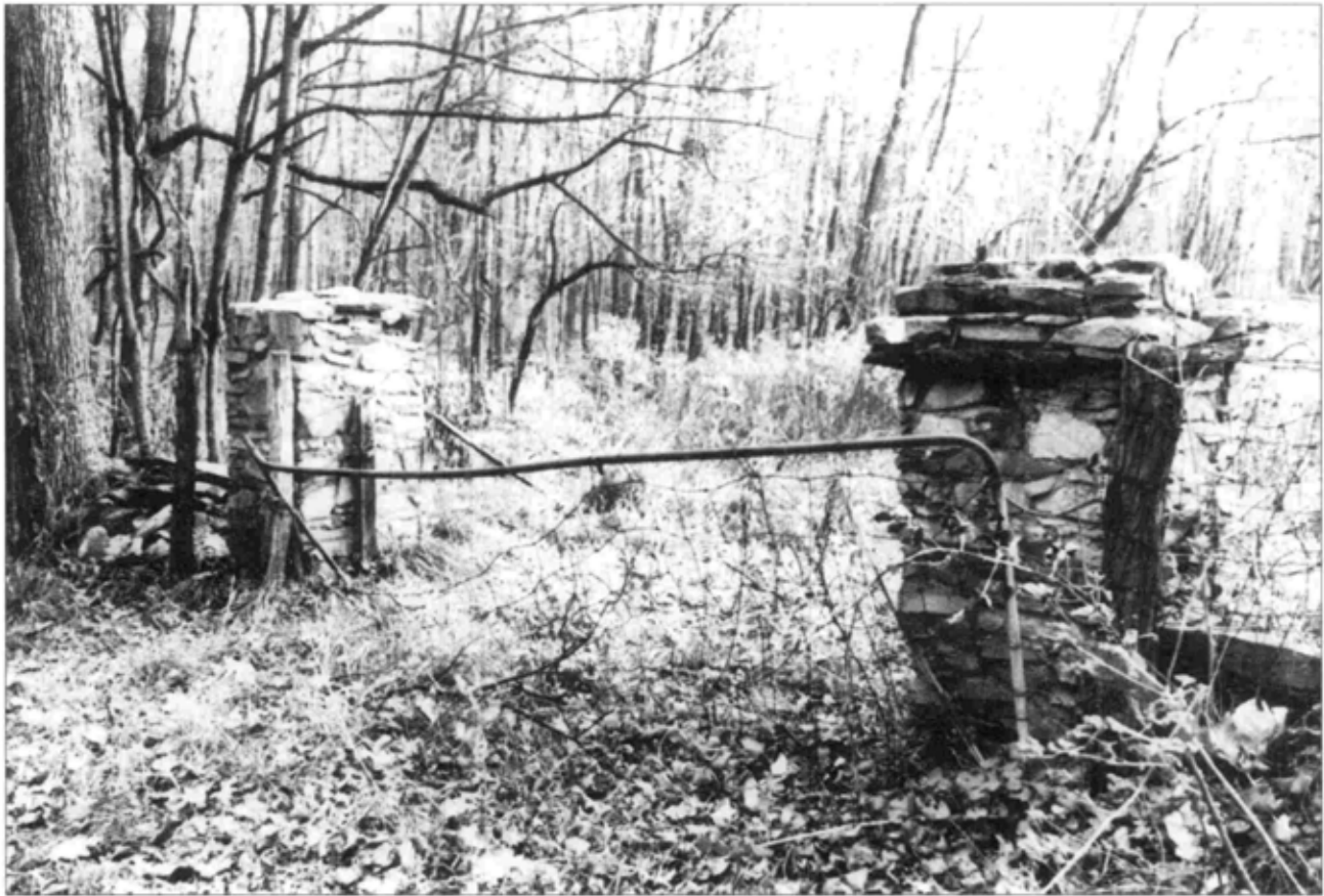
Figure 5.5. Orchard entry pillars, 1976. The stone pillars were deteriorated, one was missing its cap, and a broken metal fence was propped over the opening, replacing the former wooden slat gate. Les Hyde photo, ROVA Archives.
