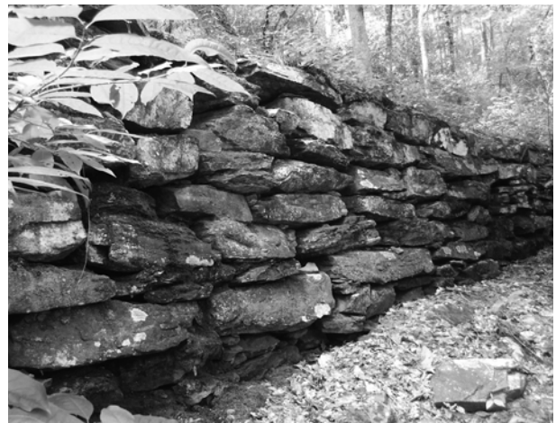
FIGURE 45. View of the retaining wall constructed for the Roswell Railroad. (Marti Gerdes, NPS-SERO-CRD, 2005)
