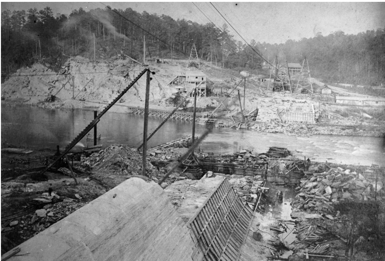
FIGURE 9. View east of construction of Morgan Falls dam and power plant, c. 1903. (Vanishing Georgia Collection, Georgia Department of Archives and History)
