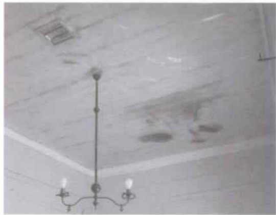
Figure 95 View of water-damaged ceiling in stranger's room. (NPS-SERO-CRS, 2001)
