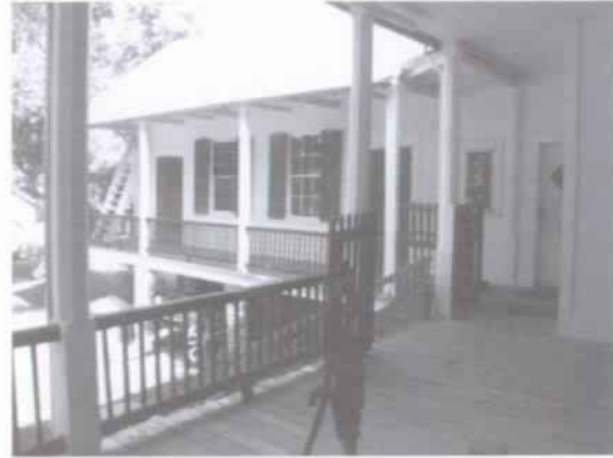
Figure 43 View to northwest on rear gallery, showing intersection with gallery on south side of kitchen wing. (NPS-SERO-CRS, 2001)
