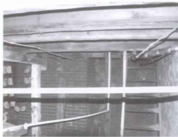
Figure 55 View north in Room 101, showing stairs to first floor, which were probably abandoned shortly after the Civil War. (NPS-SERO-CRS, 2001)
