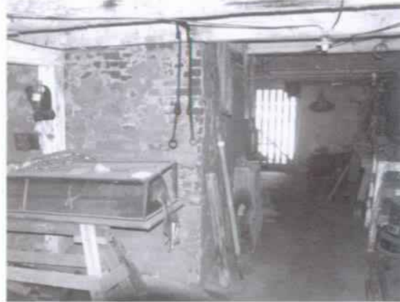
Figure 57 View to south showing connection between the two sides of Room 102. (NPS-SERO-CRS, 2001)
