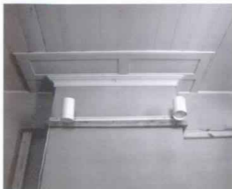
Figure 49 Board ceiling, typical of those found in most rooms on the main floor of the house. Paneling detail around chimney breast is typical of that found in 202, 205, 206, and 210, although molding details are different in each room. (NPS-SERO-CRS, 2001)
