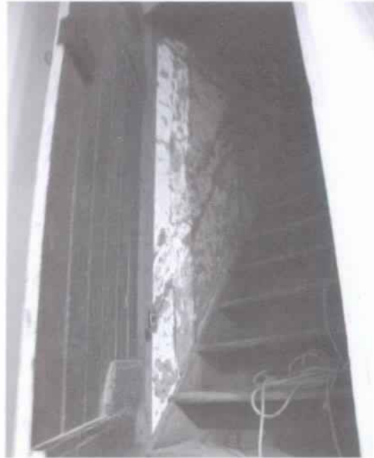
Figure 98 View of attic stairs where one of the early bousillage walls is still visible. (NPS-SERO-CRS, 2001)
