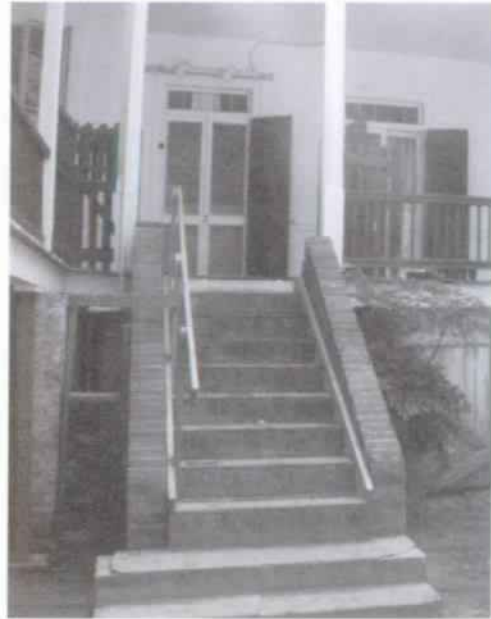
Figure 44 Brick stairs to rear gallery, shown here, and similar stairs to the south gallery replaced wooden stairs after World War II. Brick stairs to front gallery date to the nineteenth century. (NPS-SERO-CRS, 2001)
