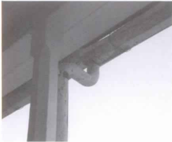
Figure 36 Typical semi-octagonal gutter and round downspouts, which date to early twentieth century. (NPS-SERO-CRS, 2001)
