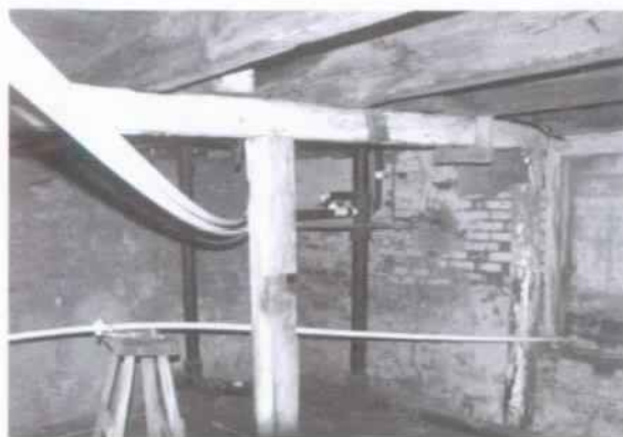
Figure 54 View southeast in Room 101, showing plumbing lines from bathroom 203. (NPS-SERO-CRS, 2001)
