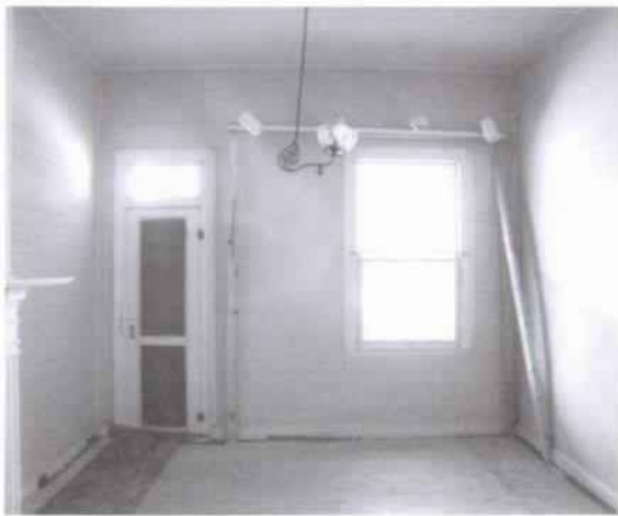
Figure 79 View north in Room 207, part of 1820s addition to original house. (NPS-SERO-CRS, 2001)
