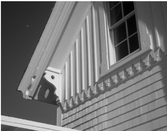
Figure C-8 Detail of north gable, showing wood shingles and board and batten siding
