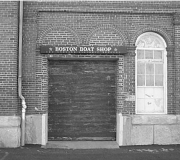
Figure 33: This coiling door in the east wall of the north wing replaced two original windows. The granite water table was also cut to make the opening. (1/15/03)
