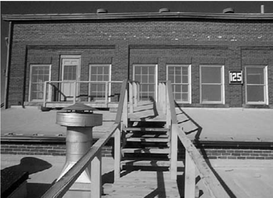
Figure 24: View of roof over the north wing. The flat metal shingles are clad with a gray liquid membrane. The wooden fire escape was rebuilt in the 1994. (1/15/03)
