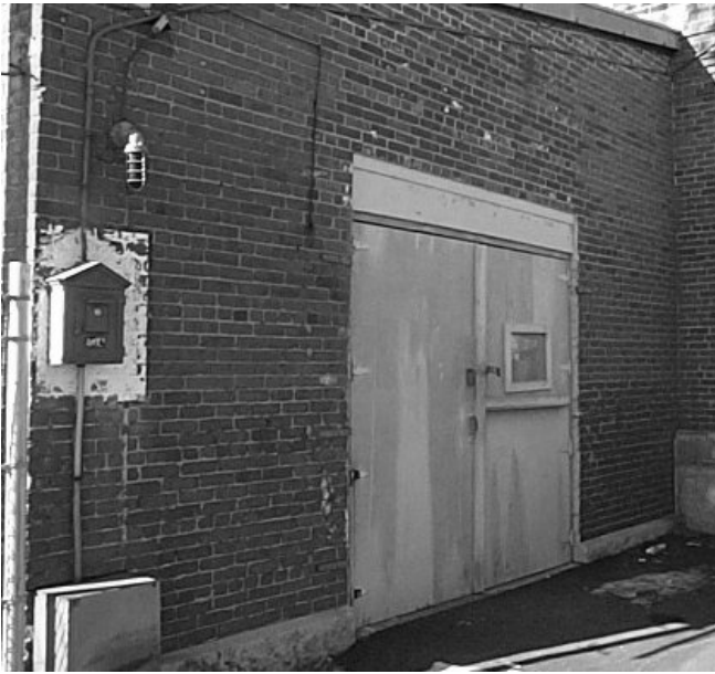
Figure 29: This hinged pair of doors in the east wall of the south wing replaced the original sliding doors. The opening was also rebuilt, with a concrete header replacing the former brick jack arch. (1/15/03)
