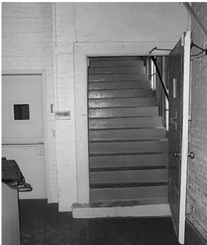
Figure 42: Stair to second floor from Room 104. The stair is original, but the freight elevator (left) replaced the original in 1939. (1/15/03)
