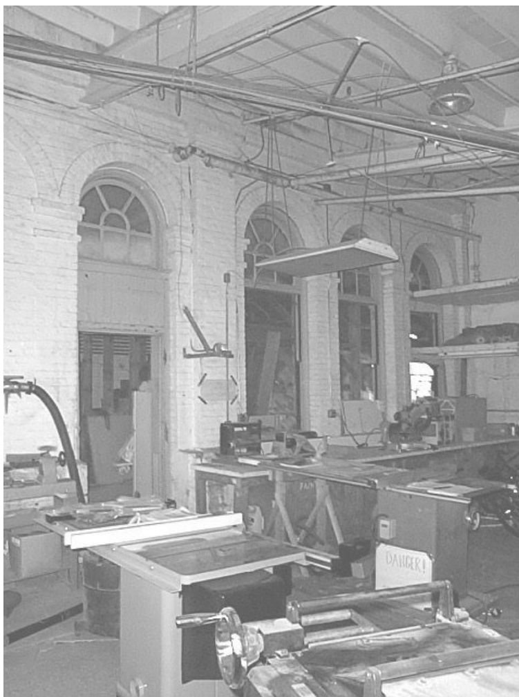
Figure 40: View of Room 106 looking south to wall that was originally the north exterior wall prior to the construction of the north extension. Note that the roof in this space is framed with wood. (1/15/03)
