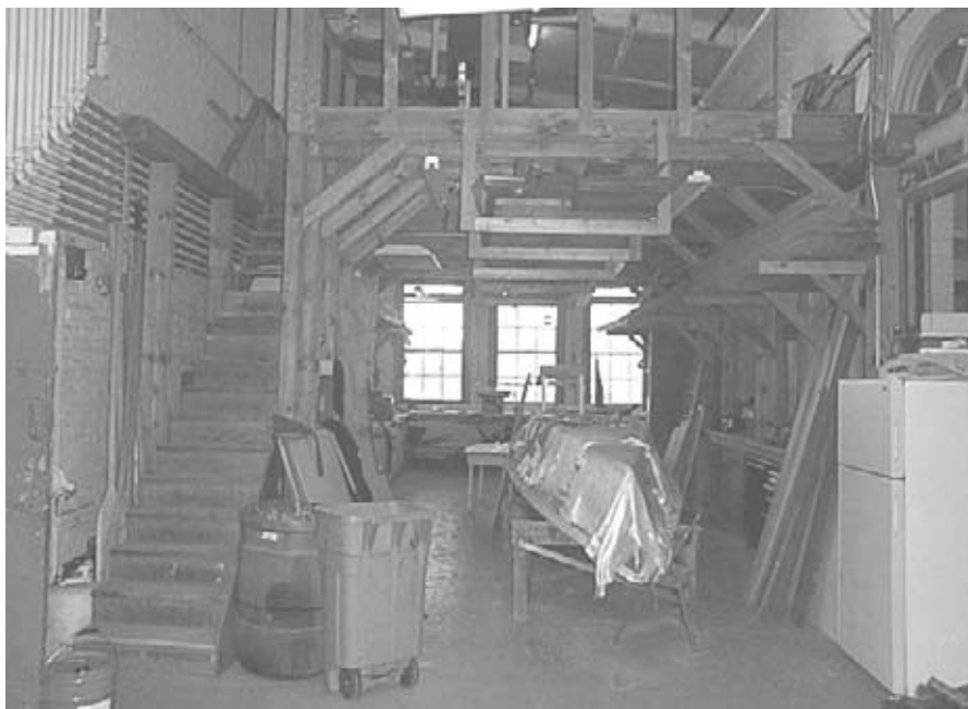
Figure 39: View looking west in north wing Room 105 showing existing wood framed loft. (1/15/03)
