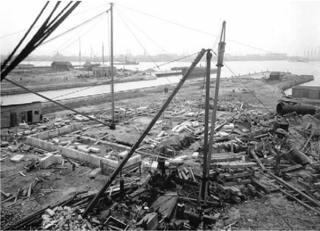
Figure 7: Foundations under construction (July 1905). Note the recently completed and flooded Drydock 2 in the background.
