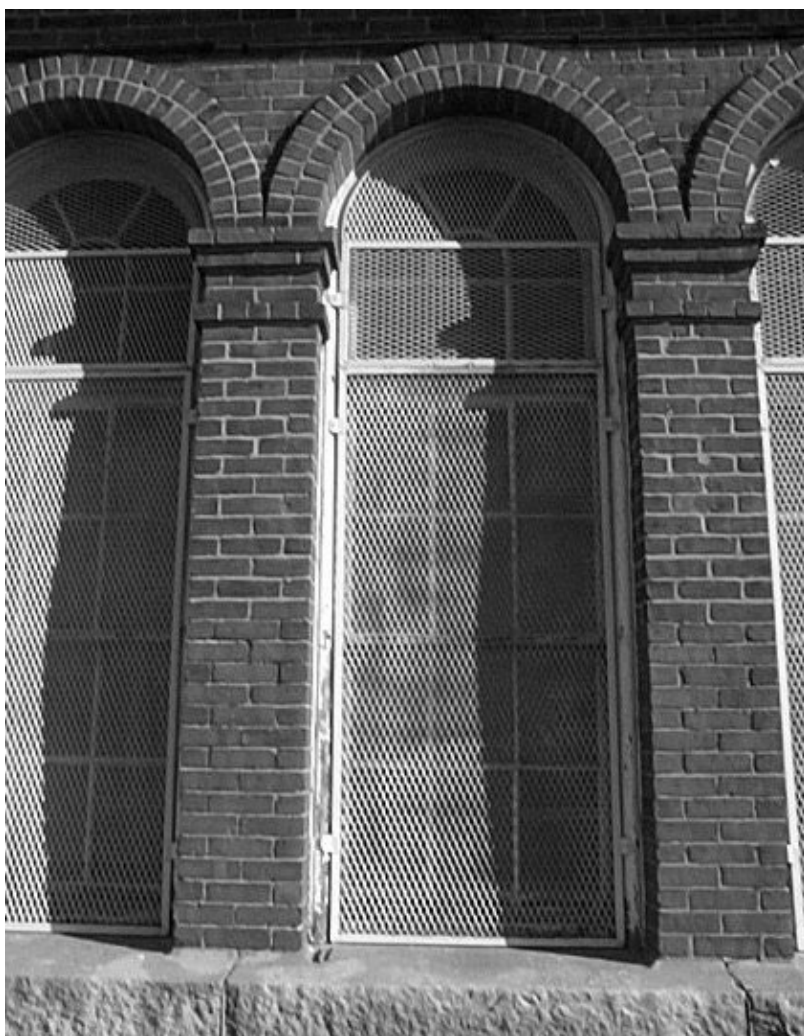
Figure 25: Typical first floor window with expanded metal security screen. (1/15/03)
