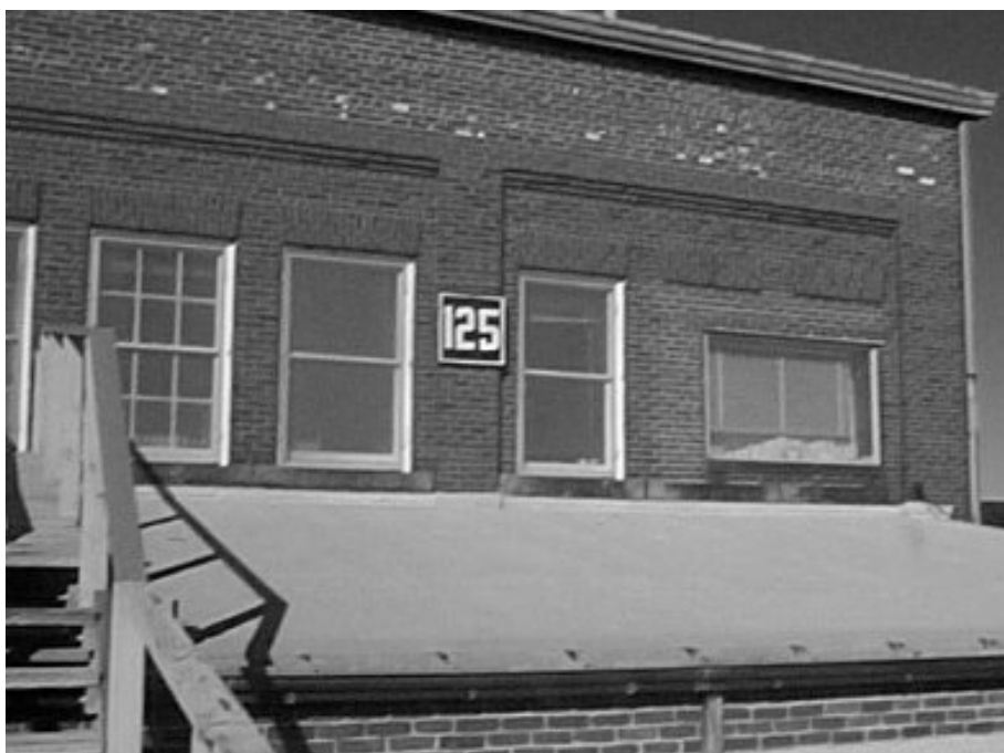
Figure 26: New windows were installed at the southeast corner of the second floor in the 1950's, including the fixed and two 1/1 double hung windows pictured here. The 6/6 window to the left is original. (1/15/03)
