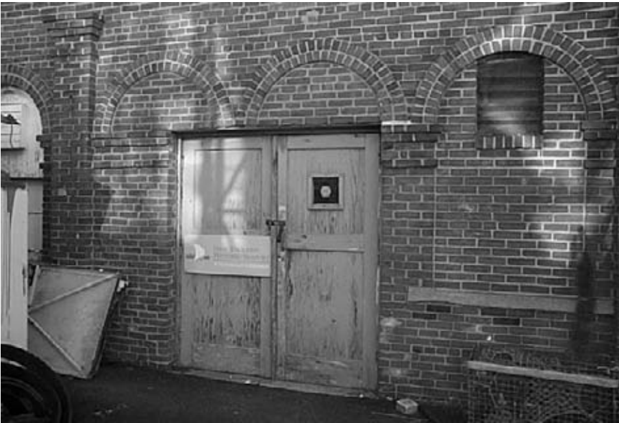
Figure 28: This pair of doors in the north wall replaced the original single door that fit into the center arch. Window openings to the left and right were filled-in. (1/15/03)
