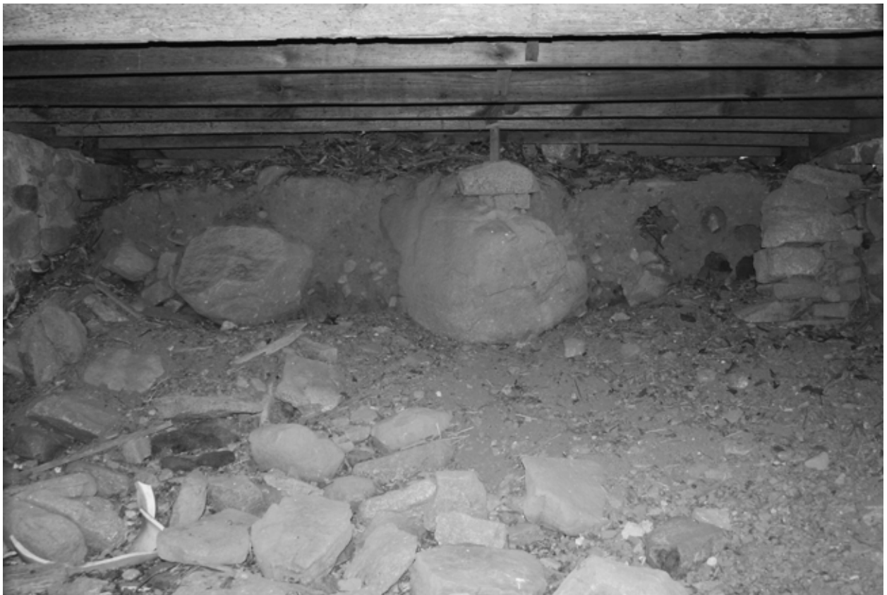
FIGURE 24. View north in cellar, with rocks from collapsed north wall in foreground. (NPS, 2005)
