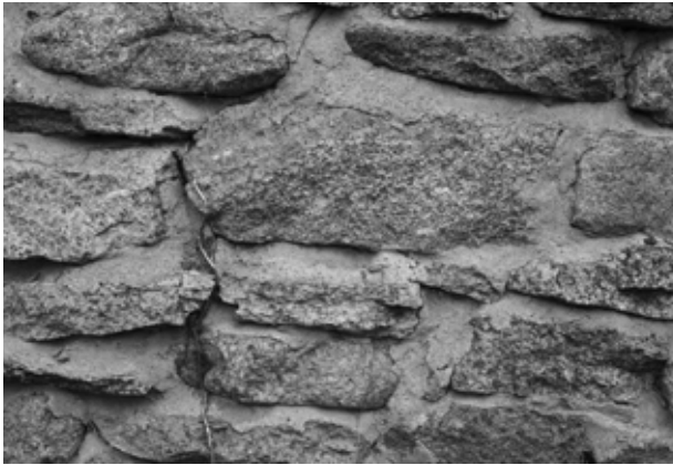
FIGURE 20. View of historic masonry near the southwest corner that has not been repointed. (NPS, 2005)
