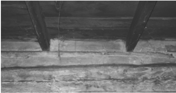
FIGURE 48. View of junction of rafters and sill plate on west side of Room 200. (NPS, 2005)
