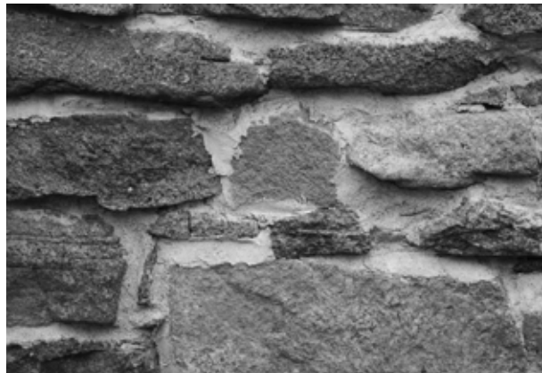
FIGURE 21. View of historic masonry that has been repointed with Portland cement. (NPS, 2005)
