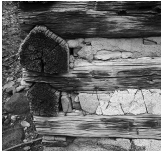
FIGURE 28. View of northwest corner of house, showing typical V-notch corners, all three generations of mortar chinking, and wire lath. (NPS, 2005)
