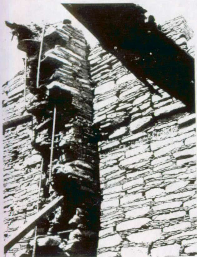
FIGURE 41. Integral members; steel in place for a narrow vertical section. The steel must be tied in securely to the cross wall at the top to provide support for the overhanging area. Some support will be required for the vertical strip of masonry as it is being laid, and until the concrete mortar has set. (Chetro Kettle Ruin, Chaco Canyon National Monument.)
