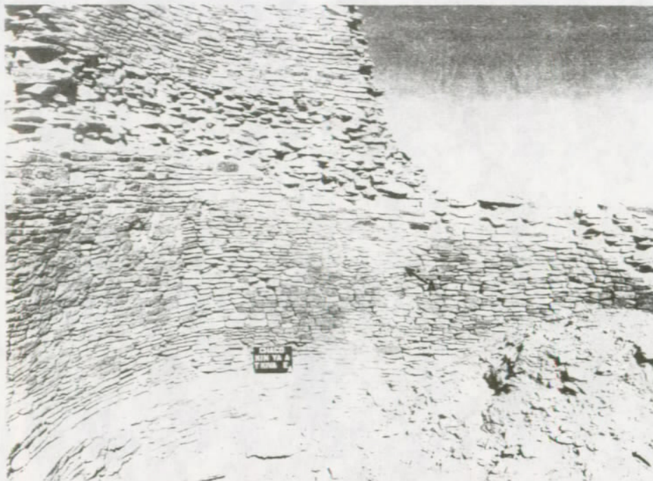
FIGURE 106. Lower portion of Tower Kiva, north and east segments, after stabilization. Offset ledges repaired, holes filled with repair masonry, facing reset (arrows A), top capped and inset core (arrow B) grouted.
