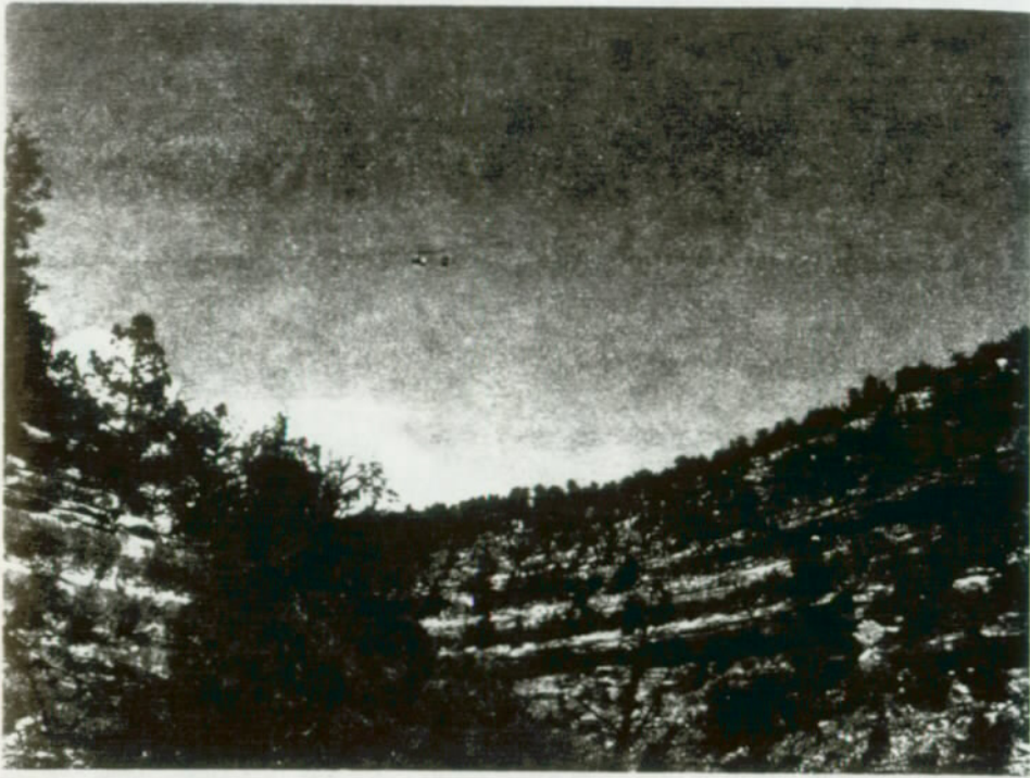
FIGURE 124. Cans of water and large bucket of stabilized mortar suspended from carrier and riding across canyon to the project. (Walnut Canyon National Monument)
