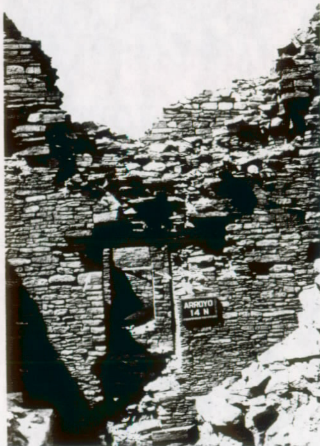
FIGURE 25. Repair at the position of the arrows will be based on a very small area in comparison with the total size of break. Every effort should be made to tie such patches securely to the existing wall. (Pueblo del Arroyo Ruin, Room 14, north wall, Chaco Canyon National Monument, N. M.)
