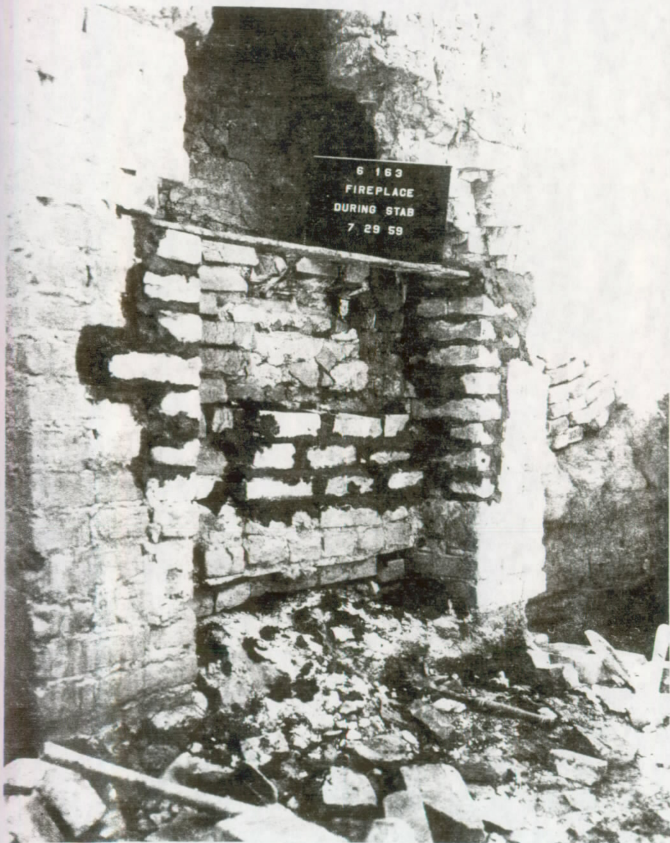
FIGURE 94. Building 6-160. Room 163. fireplace in east wall, during stabilization. Historic bricks are being reset in soil-cement mortar. Fort Union National Monument.
