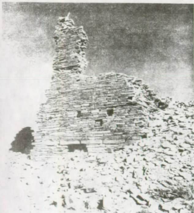
FIGURE 101. Tower Kiva, north wall exterior. Note large hole at base, and eroded insets (arrows) where second, third and fourth stories were slightly stepped back.
