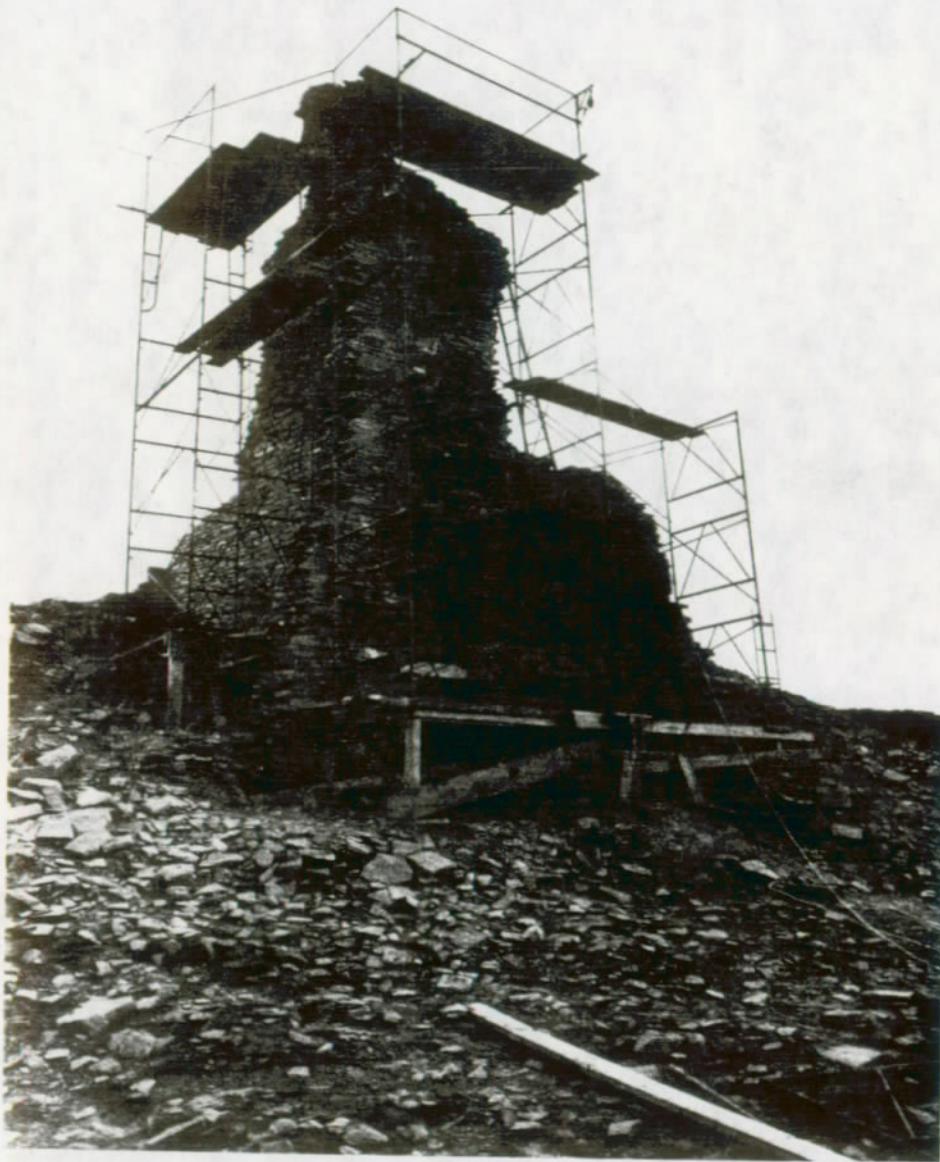
FIGURE 119. Tower Kiva. Scaffolding was anchored on firm and level bases built of heavy timbers.
