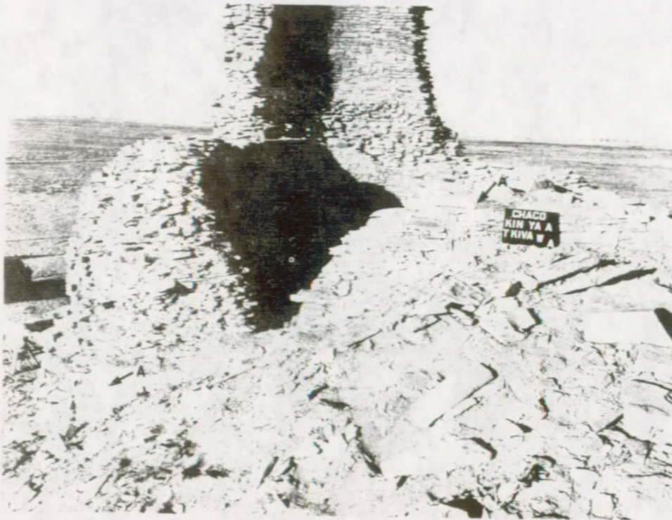
FIGURE 117. Tower Kiva, west wall. This fragmentary section of the square tower enclosing a round one was repaired by resetting the facing (arrow A), capping and grouting the thick core (B).
