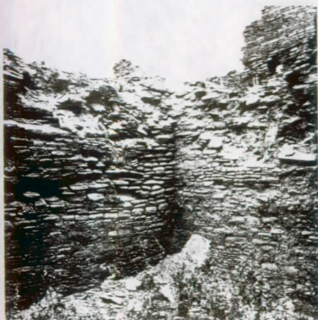
FIGURE 44. In many cases such as that depicted above it will be difficult to draw a distinction between general wall repairs and capping. This wall will have to be carried up to the level of the outside fill to prevent further washing over the top. Whatever type of mortar is used for such wall repairs, the top courses must be set in a cement mortar to provide as durable and waterproof a cap as possible. (Pueblo del Arroyo, Chaco Canyon National Monument, N.M.)
