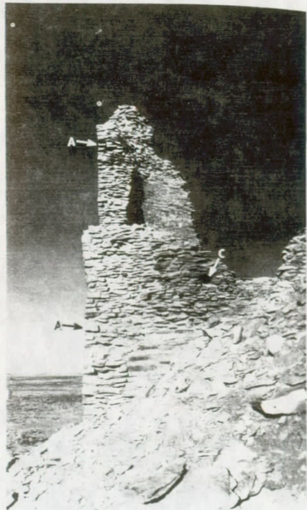
FIGURE 116. North wall stub capped (arrows A), lower portion of west wall facing reset (B), and exposed portion of thick core grouted (C).
