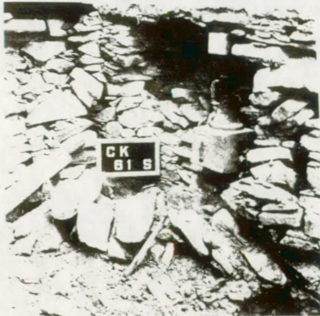
FIGURE 31. Placement of jack in line with shattered facing near the bottom of a 14-foot wall. The jack provided support while the broken area at the right was being replaced. (Chetro Kettle Ruin, Chaco Canyon National Monument, N. M.)
