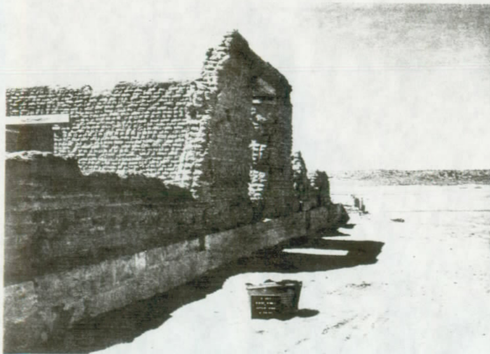
FIGURE 92. Building 3-450, Room 451, north side of north wall, after stabilization. Fort Union National Monument.
