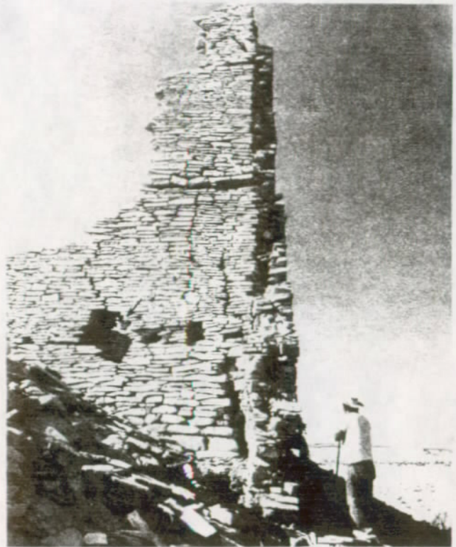
FIGURE 112. Tower Kiva, east wall exterior at juncture with north wall stub (at sign). Note the vertical cracks, eroded savino sockets (arrows) and loose, fragile spire. Portions of 4 stories are visible.
