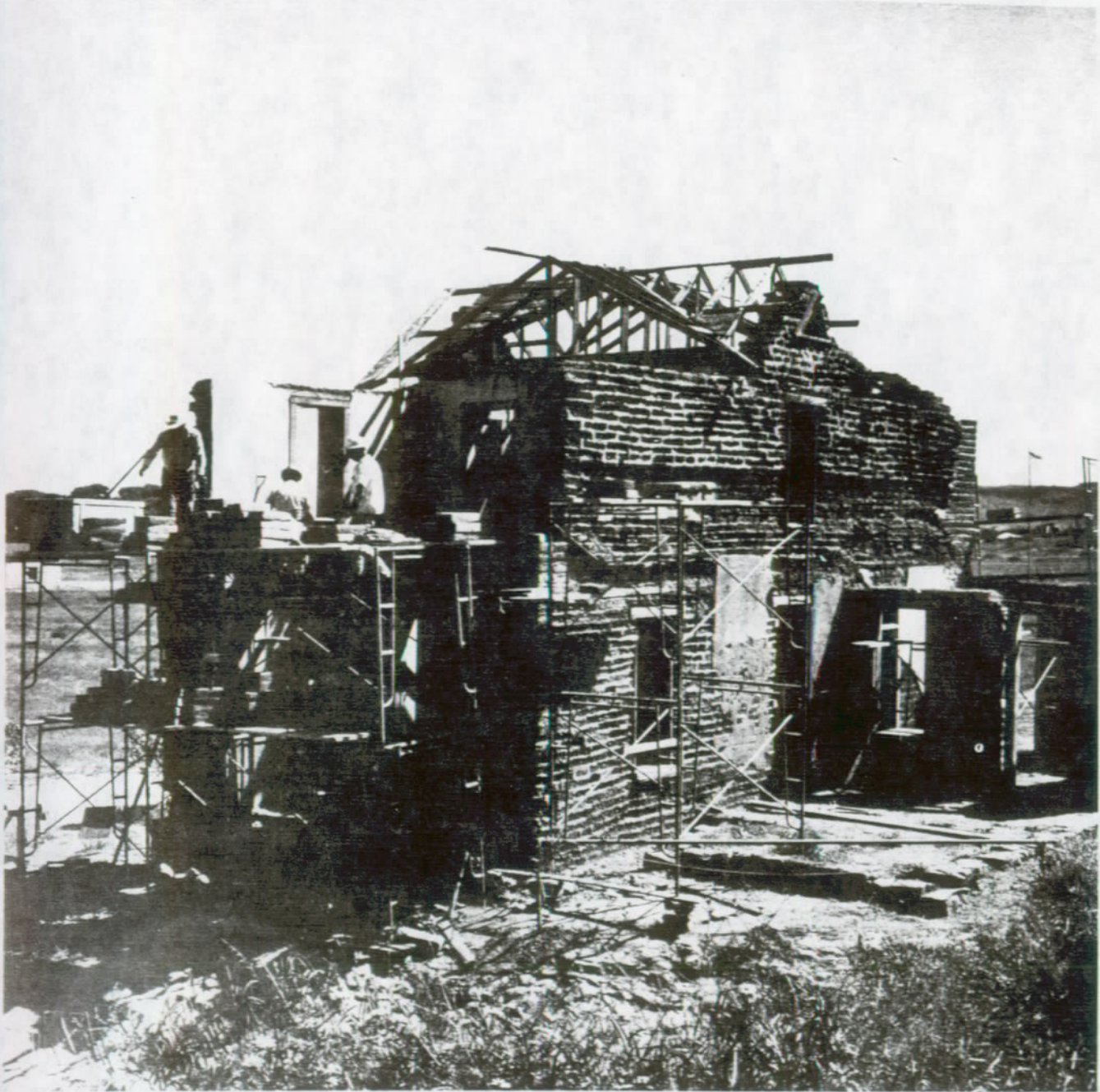
FIGURE 56. Stabilization and modified restoration in process at HB-14, shown in figure 55. Soil-cement adobes were used for repairing walls. A concealed integral bond beam was installed around the building between the first and second story levels. Concrete bearing beams were installed at roof line to support restored roof.
