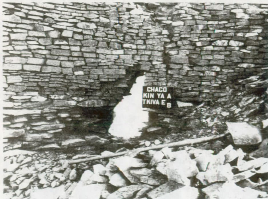
FIGURE 105. Detail of hole in Tower Kiva caused by breakdown of savino sockets. The beams for the sockets extended part way into this wall from the opposite side, and originally supported the ceiling of the adjacent room.
