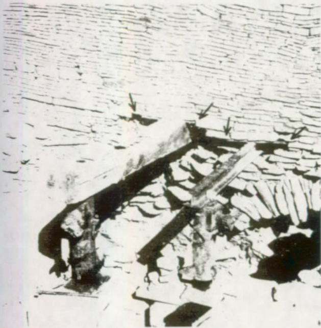
FIGURE 29. A second beam resting on jacks is placed through the wall depicted in figure 28. Arrows indicate extent of steel plates above the beam. The area of settling was reduced with upward pressure.
