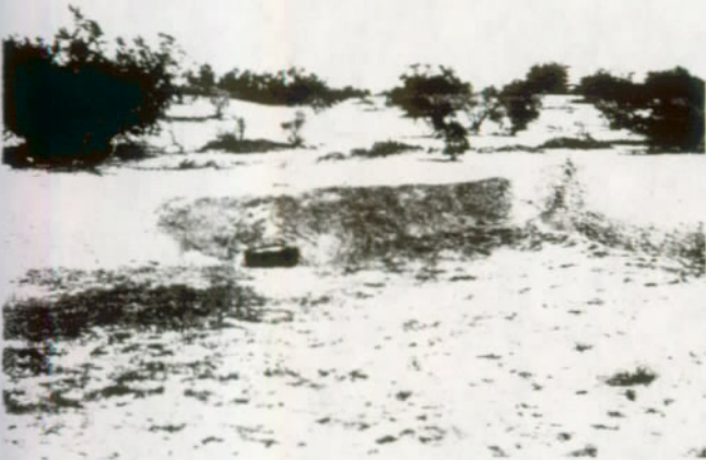
FIGURE 13. West wall of Compound A immediately after a rain. The light areas treated with silicone repelled water. The darker areas were untreated and absorbed moisture rapidly. (Casa Grande Ruins National Monument, Ariz.)
