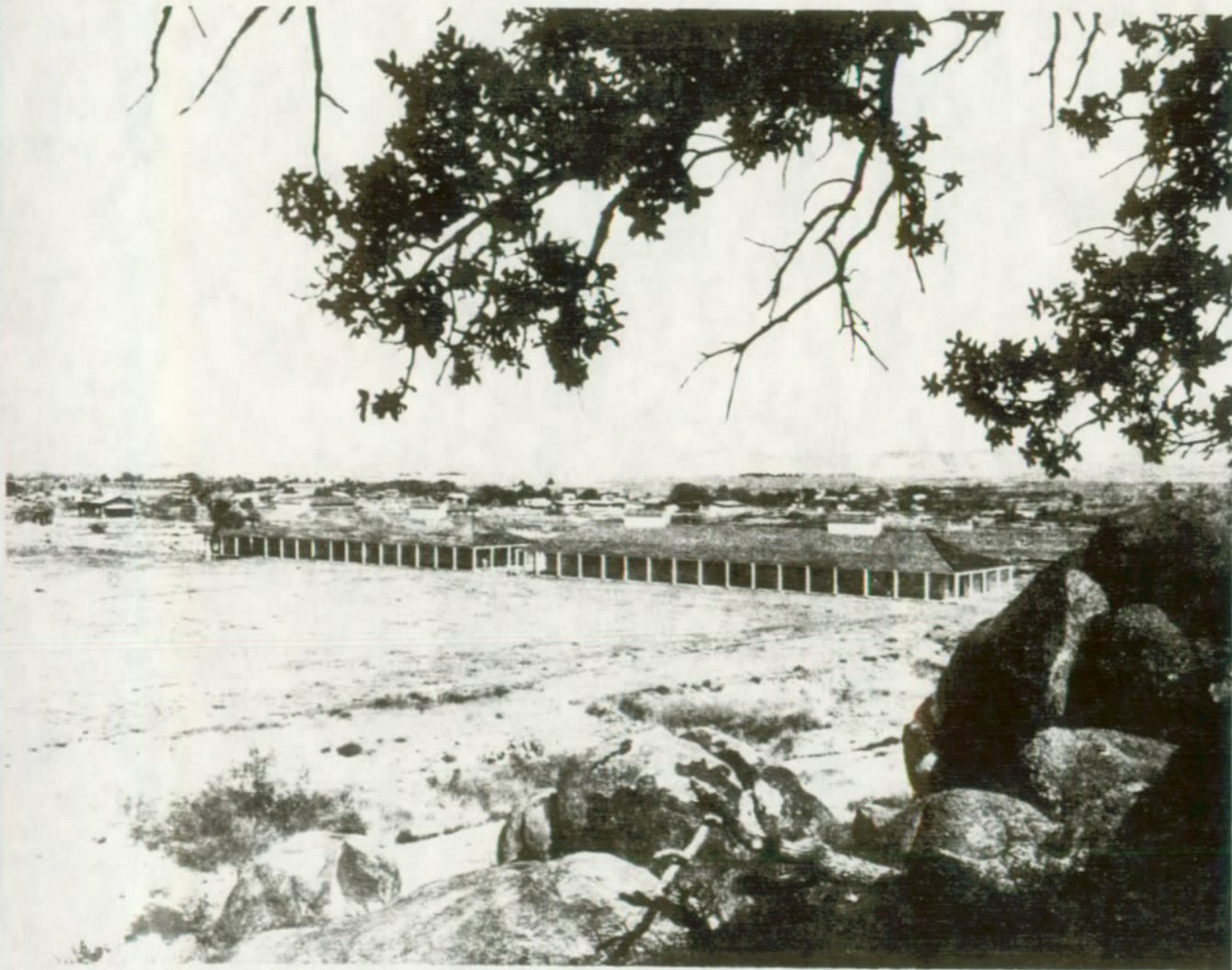
FIGURE 61. A view of the Fort Davis barracks after restoration. The ruinous shell seen in figure 60 was veneered with hand molded soil cement bricks, 4" x 4" x 12". They were made with one part portland cement (untinted), three parts unwashed sand, and three parts native soil. The bricks laid in masonry mortar with rough joints, set with spalls, were wire-brushed. Original walls were pared down where required to accommodate the veneer brick and to retain original wall dimensions and thickness. Bond beams were installed at roof line to support the restored, hipped, shingled roof. The soil cement brick walls were painted with white cement paint, although originally they were whitewashed. The building is used functionally today as the Visitor Center. Cost of the restoration: $129,000 or $12.90 per square foot.
