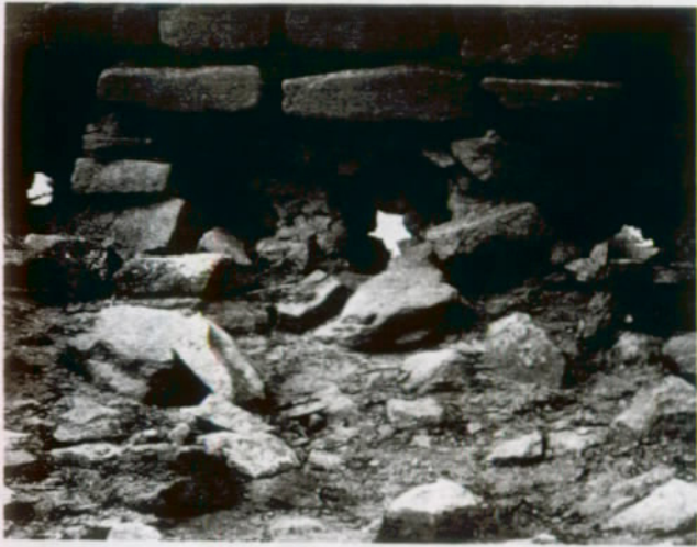
FIGURE 18. The severe undermining and basal erosion of a wall resulting from capillary moisture. If left untreated, such walls soon collapse. (West Ruin, Aztec Ruins National Monument, N. M.)
