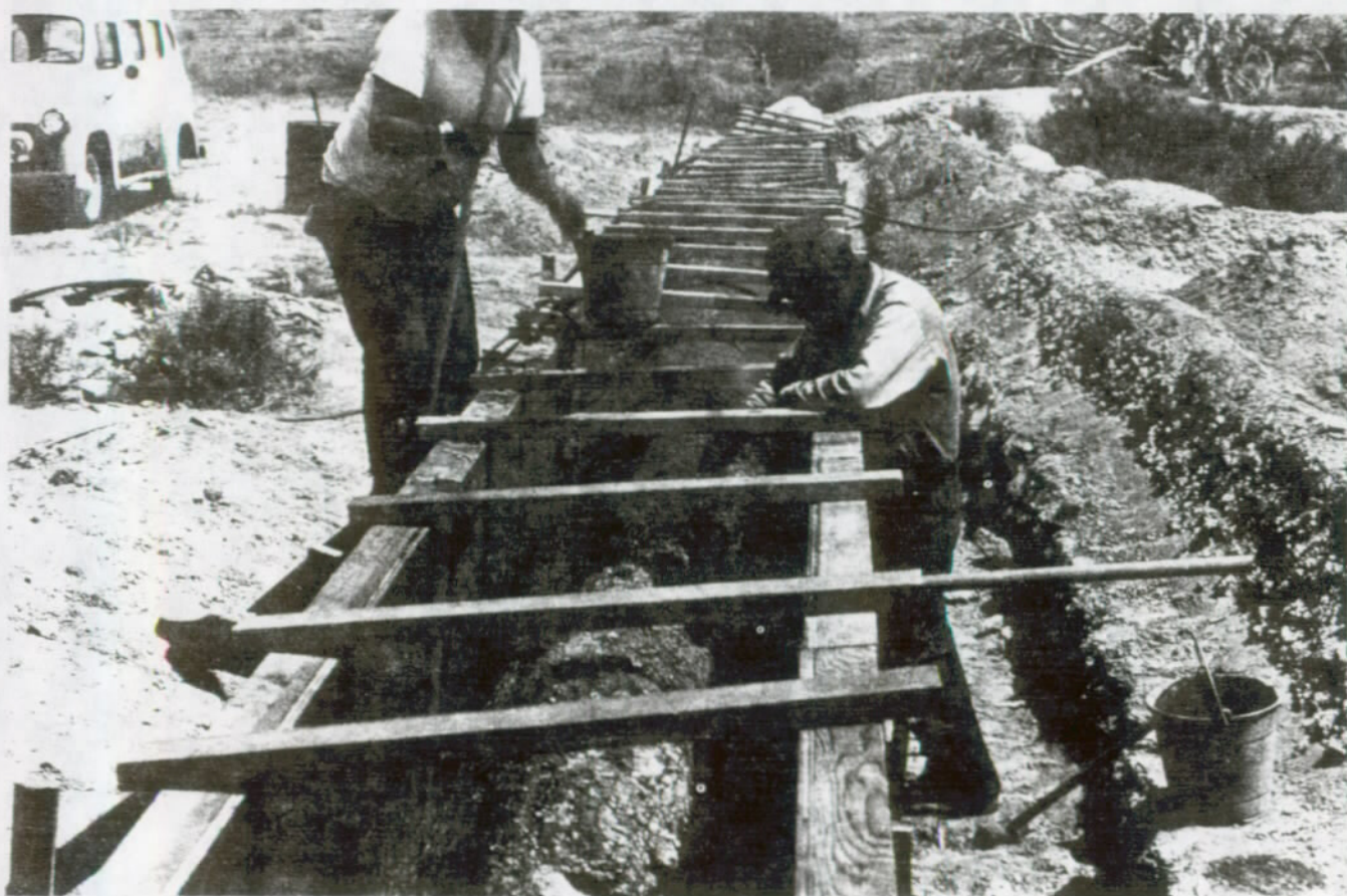
FIGURE 53. The start of placing caliche-cement mix over the wall depicted in figure 52. Note that the forms follow the irregular line of the wall.
