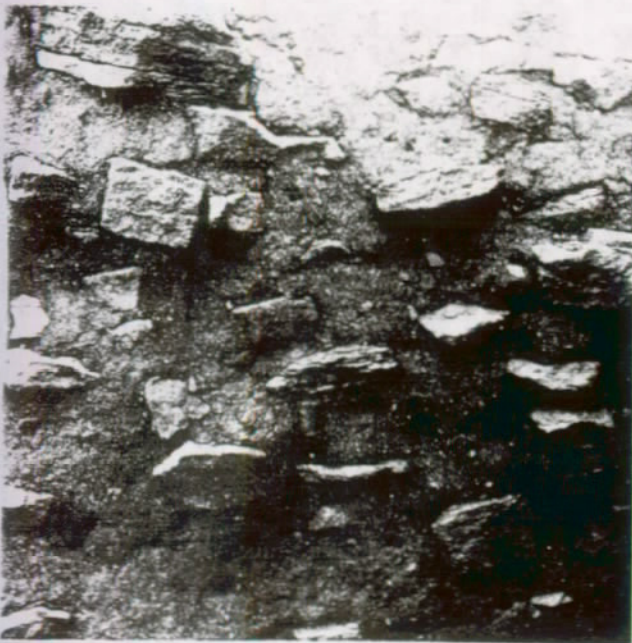
FIGURE 8. The use of heavy grouting to replace native soil between random stone; after 10 years exposure to the elements. (West Ruin, Aztec Ruins National Monument, N. M.)
