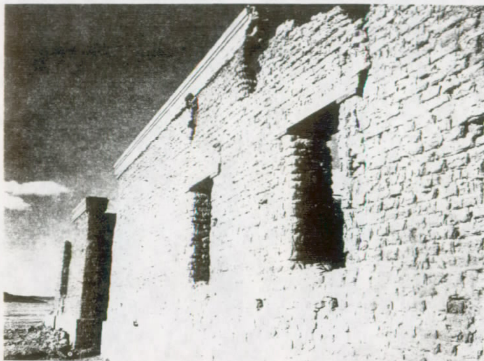
FIGURE 65. Building 3-450 (left) and building 3-440, west walls and coping, before stabilization. Fort Union National Monument.
