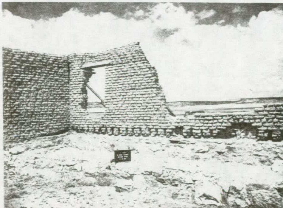
FIGURE 89. Building 3-450, Room 451, south side of north wall, before stabilization. Fort Union National Monument.
