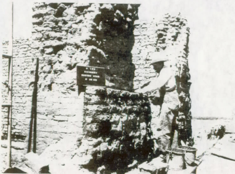
FIGURE 97. Building 6-160, Room 163, flue and chimney in east wall, during stabilization. Soil adobes are being laid to replace those that had fallen away. Fort Union National Monument.
