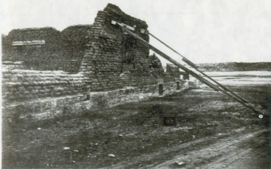
FIGURE 88. Building 3-450, Room 451, north side of north wall, before stabilization. Fort Union National Monument.
