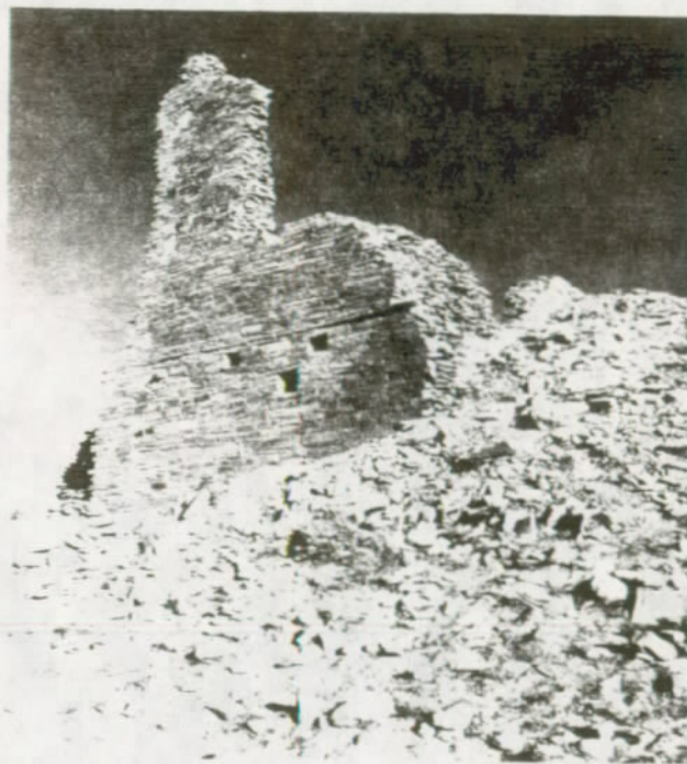
FIGURE 102. Hole at base, square openings (the two upper held beams, the lower was a ventilator) and insets repaired and wall stubs capped. Beam stub at left and two beam holes in line above (arrows) either represent reinforcing ties for kiva corner or supports for some sort of prehistoric scaffolding used in construction or a balcony.
