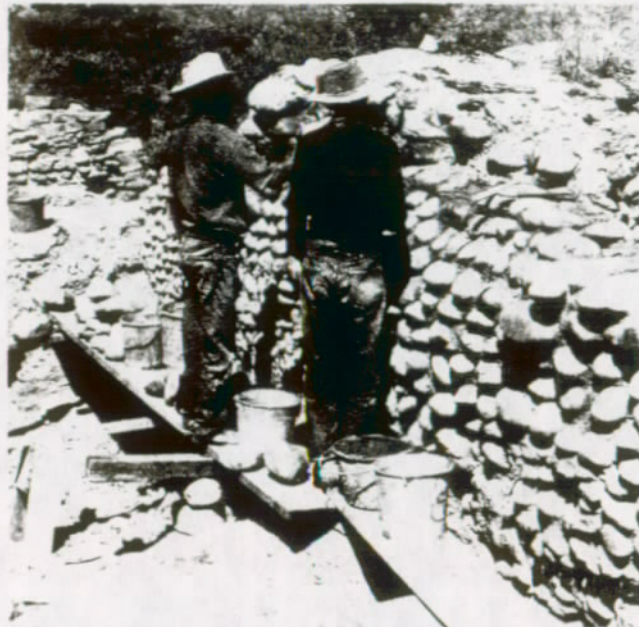
FIGURE 26. Deep grouting with soil-cement on the badly weathered face of this cobblestone wall will not change its appearance, but will halt the rapid rate of erosion. (East Ruin, Aztec Ruins National Monument, N. M.)
