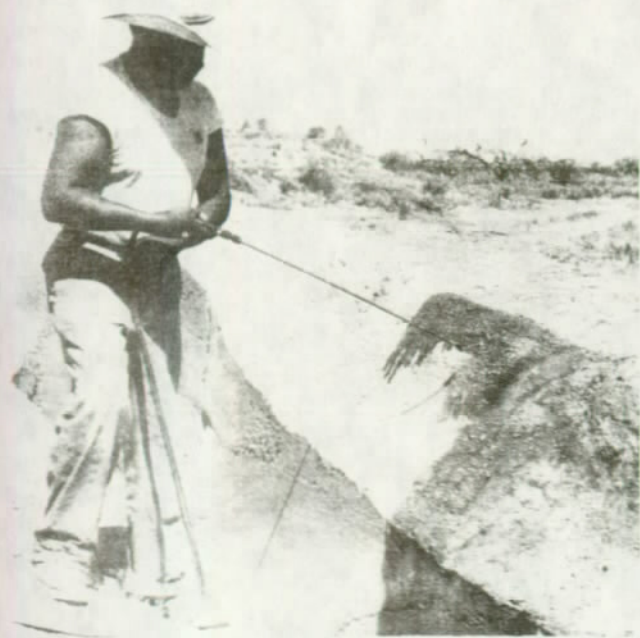
FIGURE 54. The application of a silicone water repellent. It is applied in a coarse stream, sufficient to produce a rundown of from 6 to 8 inches. (Casa Grande Ruins National Monument, Ariz.)
