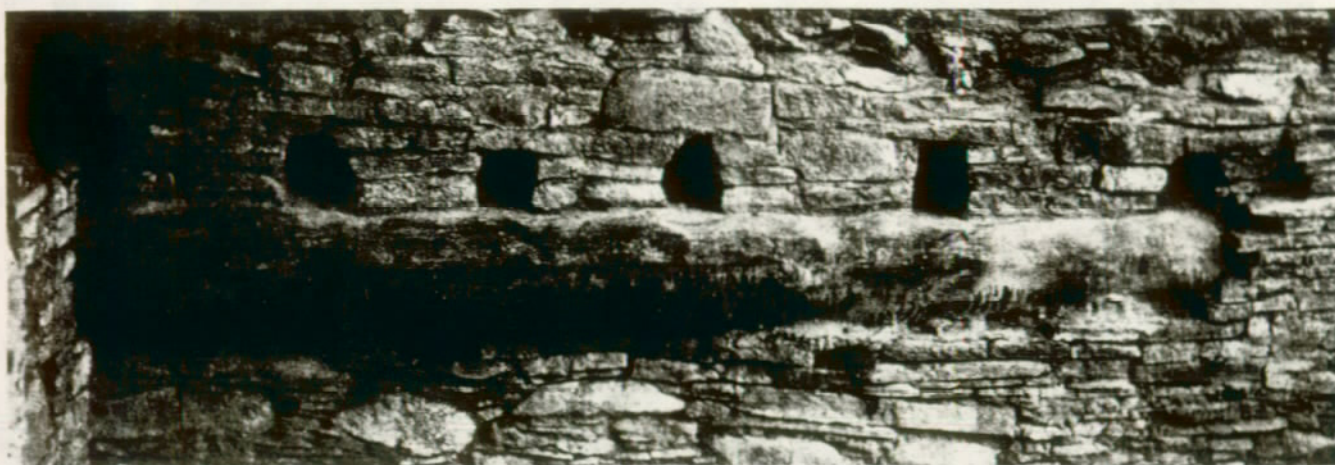
FIGURE 38. A horizontal cast log replaces the original timber which had rotted on the interior and in the embedded portions. (Chetro Kettle Ruin, Chaco Canyon National Monument, N.M.)
