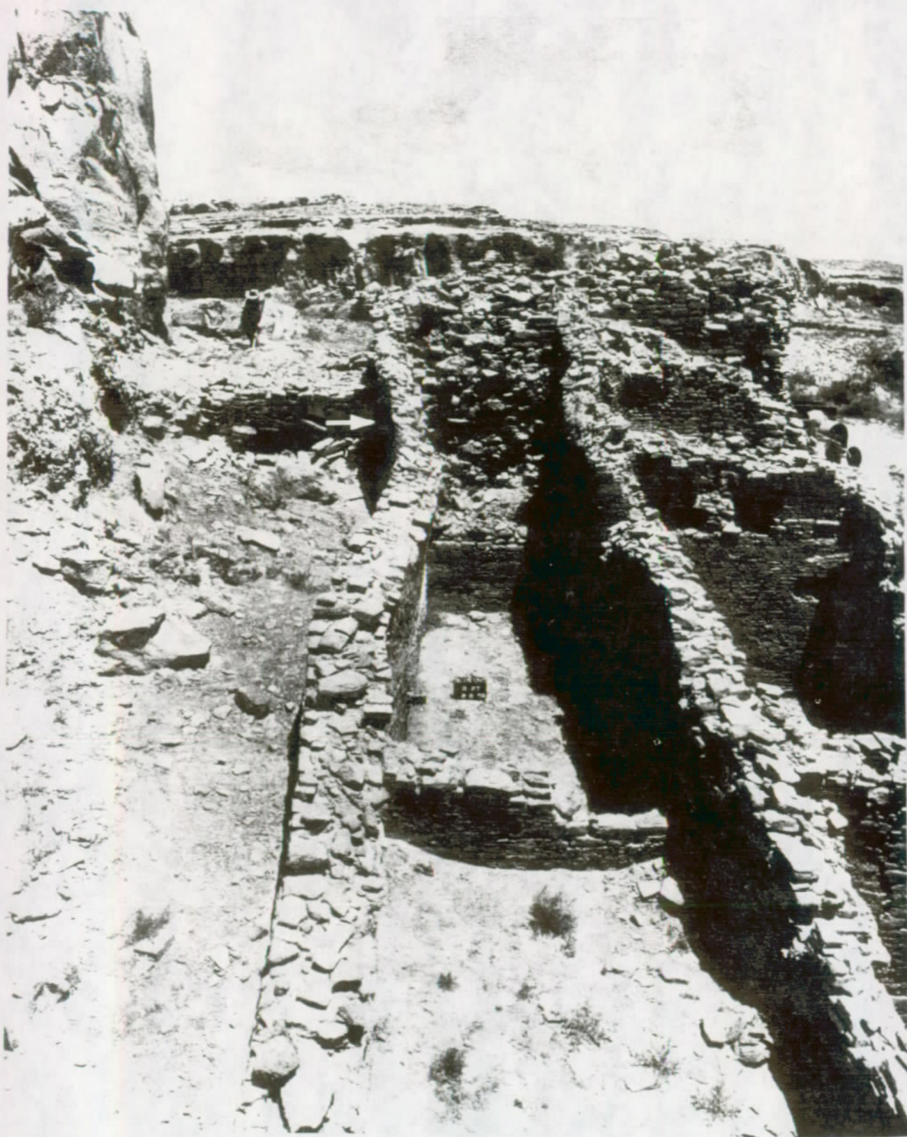
FIGURE 120. The wall between Rooms 27 and 28, Talus Unit No. 1, was distorted and pushed out of line by pressure of fill, often damp, at left. Arrow shows direction of force. The purpose of the stabilization was to strengthen the wall against the pressure.
