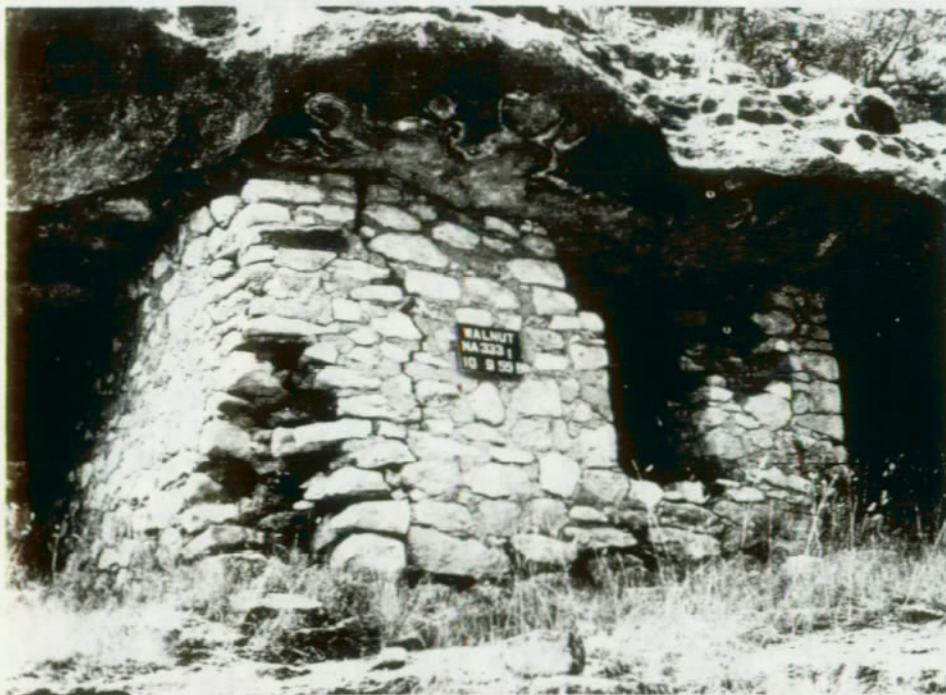
FIGURE 125. Room 1, east exposure, before replacement of fallen corner. (Walnut Canyon National Monument)
