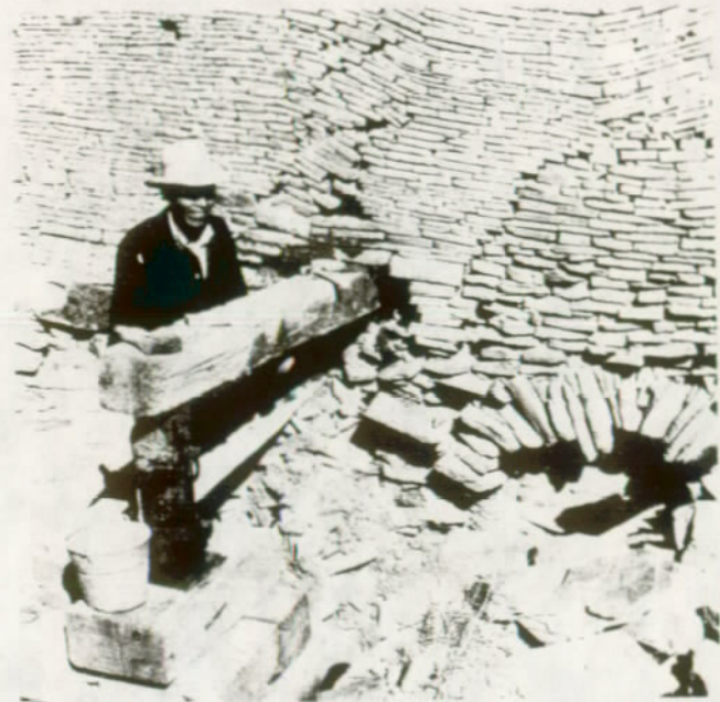
FIGURE 28. The temporary support of a heavy wall with timber. The arch at lower right was constructed in the 1920's as a repair measure. The first step in stabilization involved the placing of a beam through a hole adjacent to the arch. Not of aboriginal origin, the arch was subsequently removed. (Room 1, Chetro Kettle Ruin, Chaco Canyon National Monument, N. M.)
