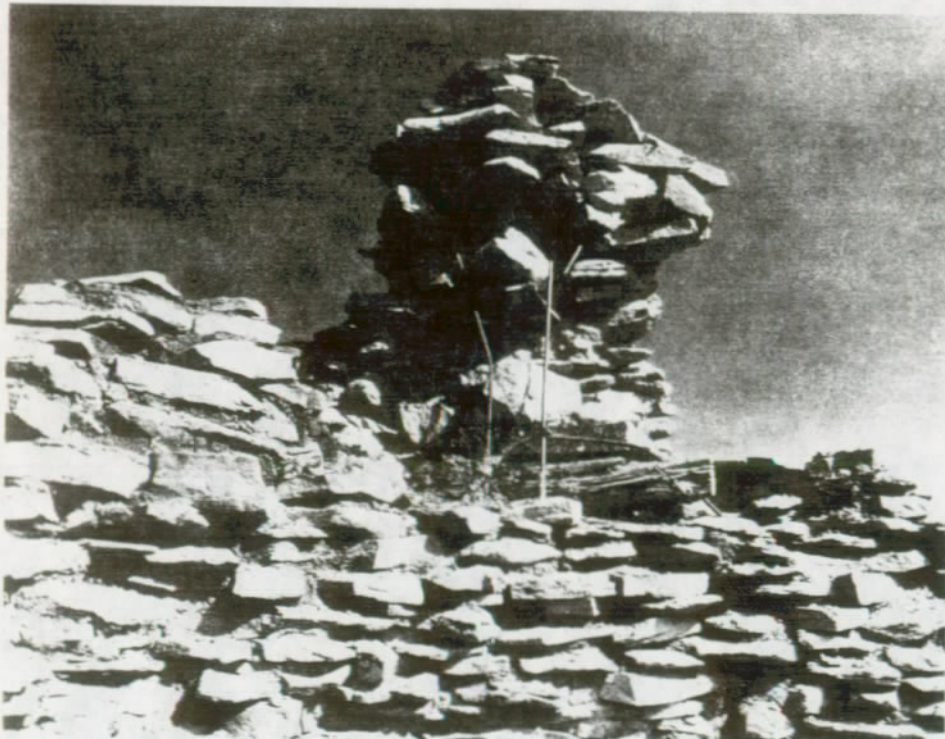
FIGURE 110. Integral members in the form of a T were installed in this top fragment of core masonry after the lower wall section had been strengthened to that point.
