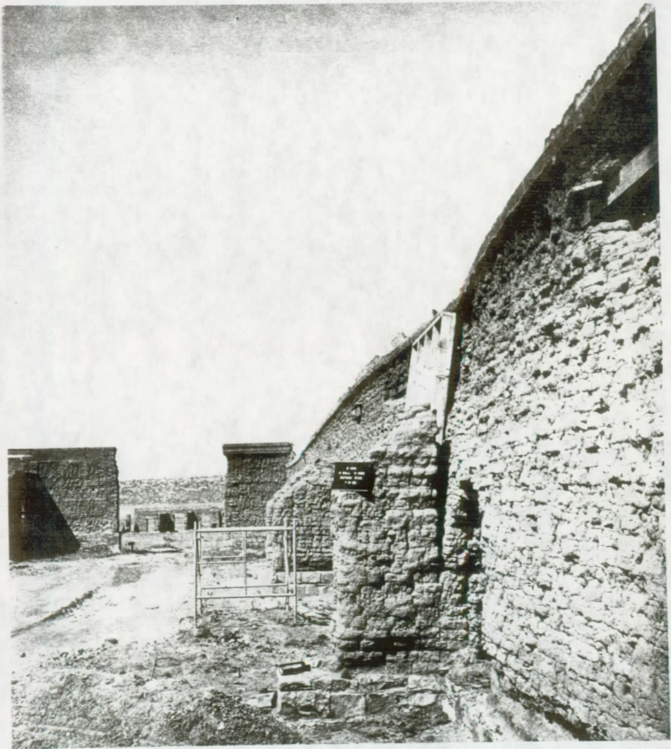
FIGURE 77. Building 3-450, Room 451, south side of south wall, before stabilization. Fort Union National Monument.
