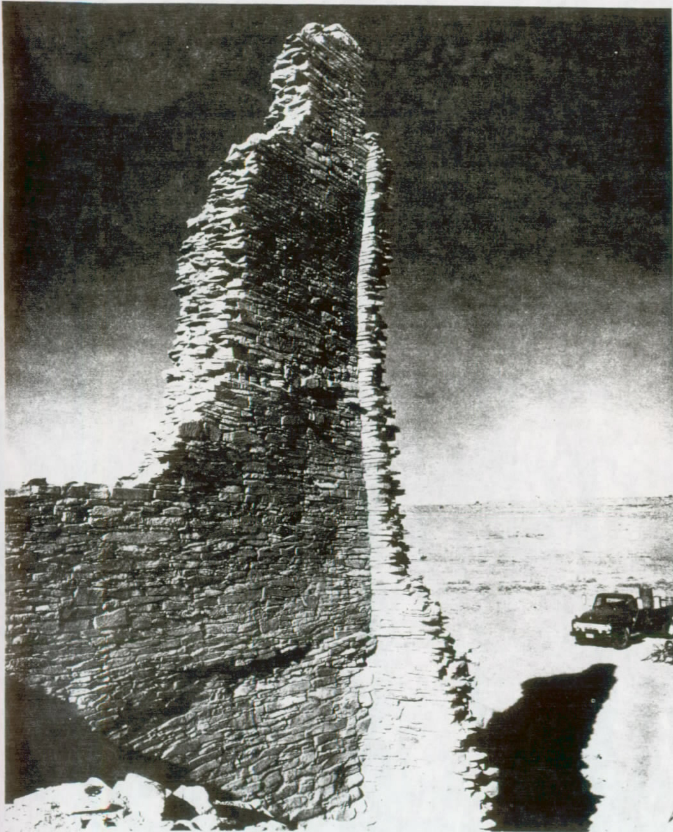
FIGURE 114. View of Tower Kiva showing north wall stub buttressed, cracks repaired, savino sockets re-molded, and facing grouted.
