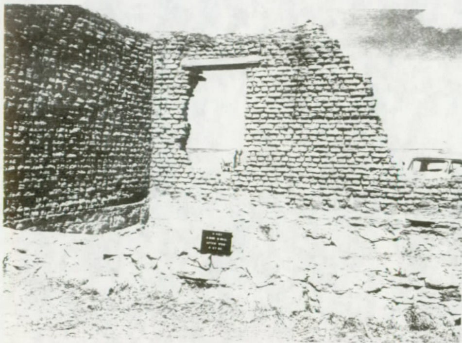
FIGURE 91. Building 3-450, Room 451, south side of north wall, after stabilization. Fort Union National Monument.
