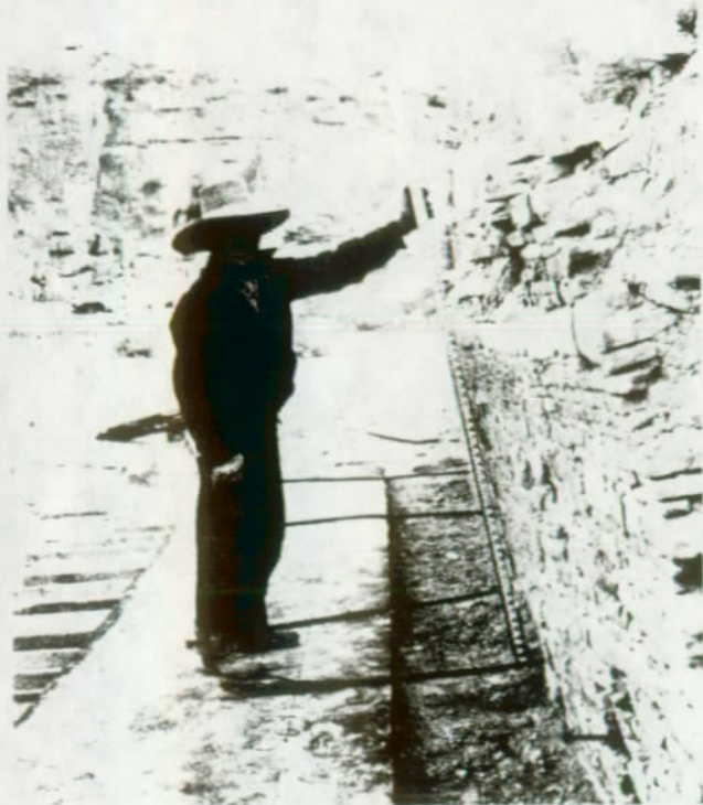
FIGURE 33. Beginning realignment. Cables have been placed through the base of the wall to be tied to the jacks. Note bolt, lower right, for holding frame against wall. (Pueblo Bonito, Chaco Canyon National Monument, N. M.)
