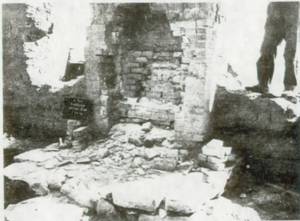
FIGURE 93. Building 6-160, Room 163, fireplace in east wall, before stabilization. Fort Union National Monument.
