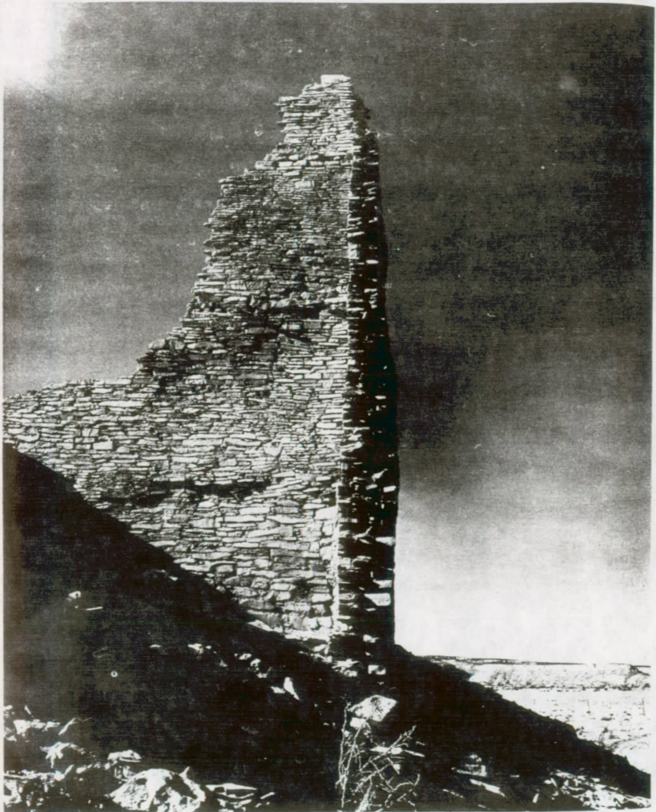
FIGURE 113. View of Tower Kiva showing vertical cap.
