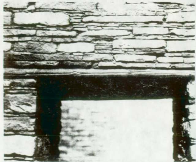
FIGURE 37. The cast concrete lintels have the same appearance as the originals from which they were cast. (Chetro Kettle Ruin, Chaco Canyon National Monument, N. M.)
