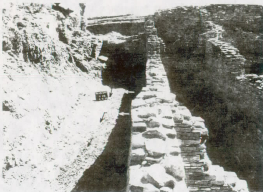
FIGURE 123. This wall in Talus Unit No. 1 has been pulled back into line; the capping is straightened up. The concrete beam dug into Room 28 is covered and the surface of this room (arrows) is graded to carry surface runoff away from the damaged wall.
