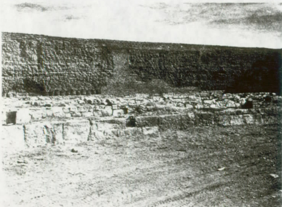
FIGURE 85. Building 3-450, Room 451, north side of south wall, after stabilization. Fort Union National Monument.
