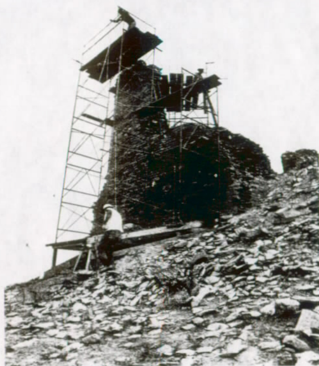
FIGURE 42. Reinforced integral members are important in the stabilization of spirelike structures such as this at the Tower Kiva, Kin Ya-a Ruin, Chaco Canyon National Monument, N. M. Considerable strength must be added without serious or objectionable alterations of the original profile.
