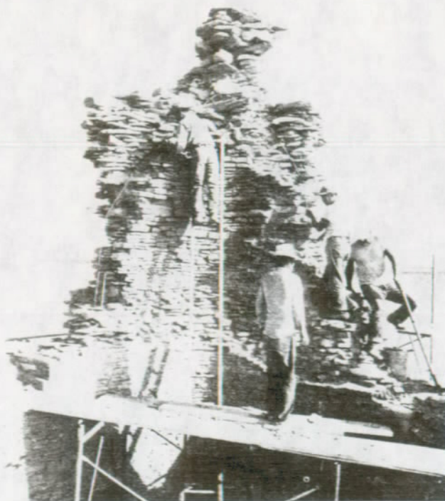
FIGURE 107. Tower Kiva, interior northeast corner, during installation of integral members to strengthen the highest wall section.
