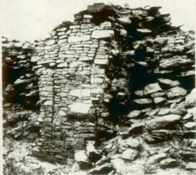
FIGURE 46. A good deal of repair masonry must be laid to fill breaks and support undercut areas in this wall at Pueblo del Arroyo. Some support must also be provided for the embedded timbers. Soil or masonry cement mortars may be used for the major part of this work. The upper courses however must be laid in concrete mortar as capping to halt further washing from the top. In this example, damage was started by surface water from adjacent, unexcavated fill and every effort should be made to prevent erosion.
