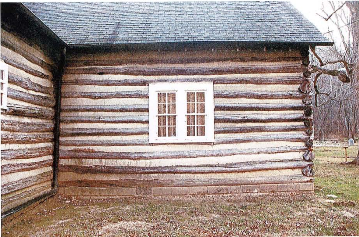
Figure 5 The bow in the bottom logs and the wide band of chinking indicates that severe deterioration is present at the base of this wall.
