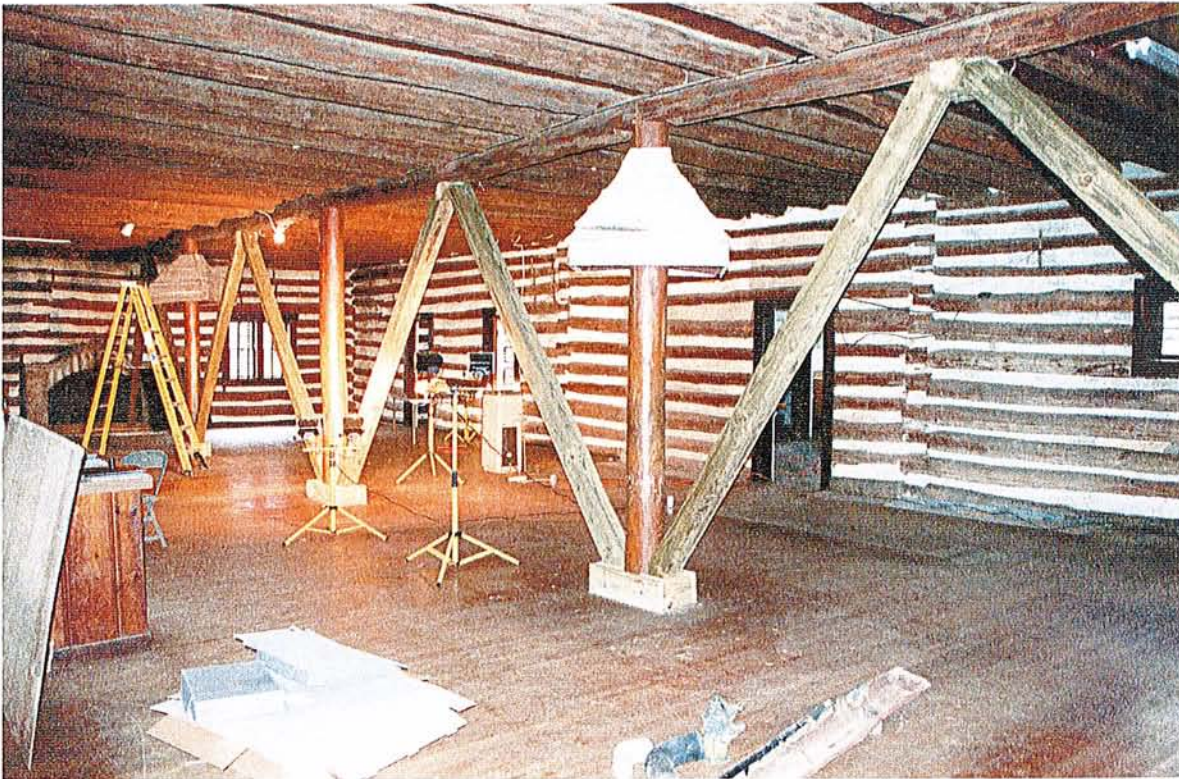
Figure 9 Large diagonal 6 x 6 braces were added to reinforce the second floor log beams.
