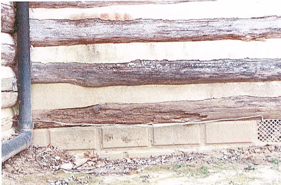
Figure 6 Stains and cracks in the chinking are clues to possible wood deterioration.
