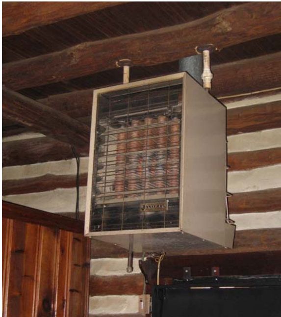
Figure C-38 Unit heater in Room 102
