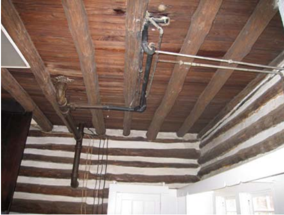
Figure C-30 Ceiling of the kitchen, showing exposed plumbing
