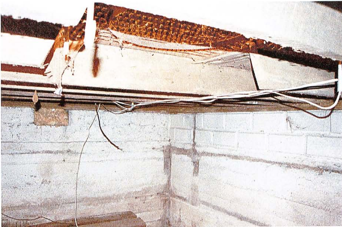
Figure 7 This vent was added without a header provided where the floor joists were cut.
