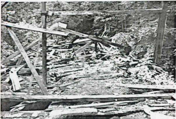
Figure 38 Headhouse Existing Condition Photo: Structural Detail. Collapse of roof structure. View toward mine opening. 1986. Photo courtesy of West Virginia University.
