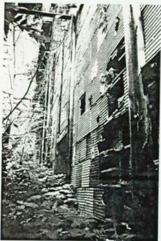
Figure 29 Powerhouse Existing Condition Photo: Structural detail. Hollow clay tile wall between compressor room and old boiler room looking towards building east. July 1996. NPS photo.
