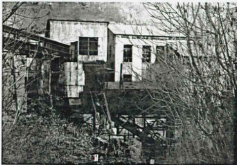
Figure 18 Coal Tipple Existing Condition Photo: West elevation. Rusted roof sheathing and broken windows. Note monitor conveyor at upper left.
