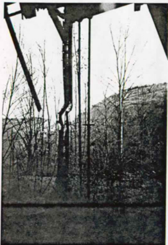
Figure 22 Coal Tippie Existing Condition Structural Detail: Column 4E column failure due to weak axis buckling and broken cross bracing. Two temporary pipe columns to the right. Nov. 1996. NPS photo.
