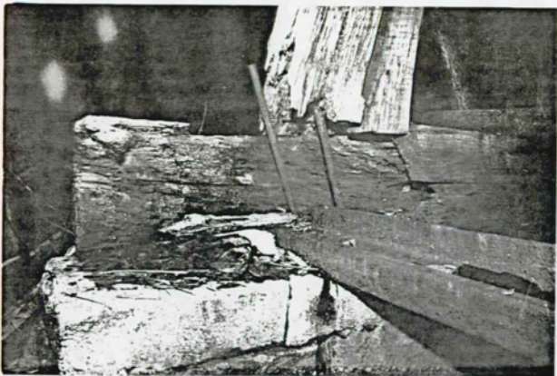
Figure 39 Headhouse Existing Condition Photo: Structural detail. Typical column/sill joint showing severe rotting of members. 1986. Photo courtesy of West Virginia University.
