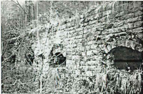
Figure 31 Coke Ovens Existing Condition Photo: Semicircular arched opening with fallen voussoirs. Vegetation and lack of historic oven doors is accelerating arch failure.
