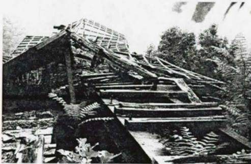
Figure 34 Headhouse Existing Condition Photo: Remains of 1990 stabilization efforts and reroofing.
