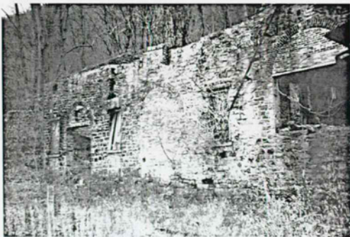
Figure 25 Powerhouse Existing Condition Photo: East elevation of boiler room. Note crumbling upper wall surfaces, brick infill, deteriorated wall base and sill at right. Nov. 1996. NPS photo.
