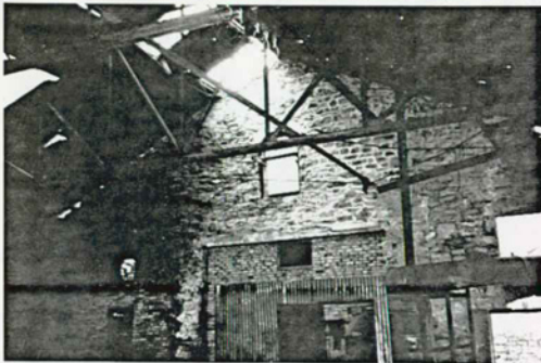
Figure 28 Powerhouse Existing Condition Photo: Structural detail. Interior of compressor room. Roof damage visible, view towards north. Noted later brick infill at base of wall. Nov. 1996. NPS photo.
