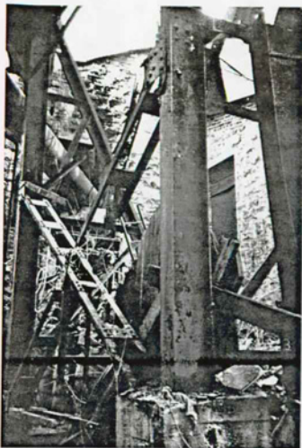
Figure 21 Coal Tippie Existing Condition Structural Detail: Failed cross-bracing between columns 7A and 8A. Note powerhouse in background.
