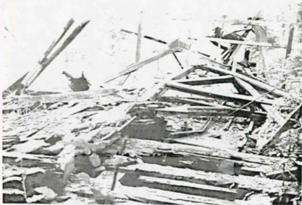
Figure 36 Headhouse Existing Condition Photo: Collapse of roof structure. View toward river. 1986. Photo courtesy of West Virginia University.
