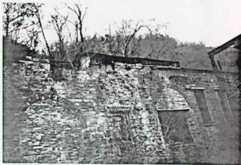
Figure 23 Powerhouse Existing Condition Photo: East elevation. Roof missing over boiler room (to left). November 1996. NPS photo.
