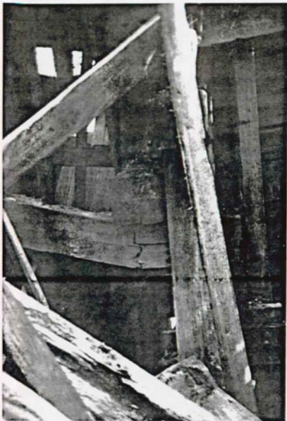
Figure 42 Headhouse Existing Condition Photo: Structural detail. Flexural failure of interior beam on Bent G. 1986. Photo courtesy of West Virginia University.
