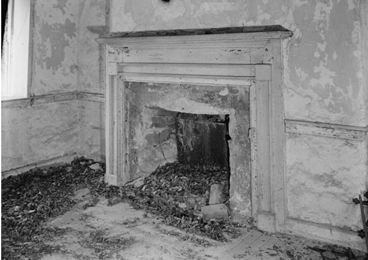
Illustration 17 Fireplace in house at Lock No. 27, 1959 photograph. Photograph by Jack E. Boucher. From Historic American Buildings Survey Files.
