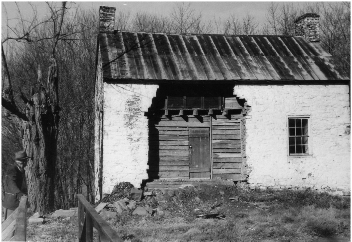
Illustration 14 House at Lock No. 27 showing dilapidated condition of structure, Dec. 1959 photograph. Photograph by Jack E. Boucher. From Historic American Buildings Survey Files.
