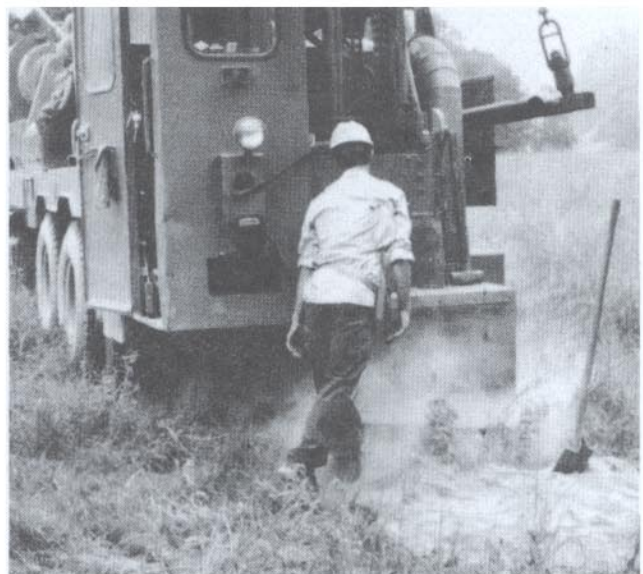
Rock driller working without respiratory protection on a mobile rig.
