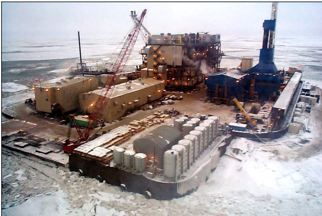
BP's Northstar production island in 39 feet of water off Prudhoe Bay, Alaska. (Photo courtesy of David Dickins, DF Dickins Associates, Ltd.)
