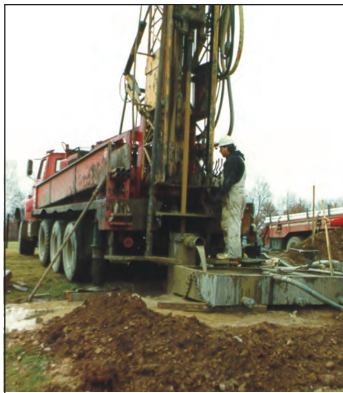
Figure 1. A new well being drilled in Oakland County. Over 3,000 new drinking-water wells are drilled each year in Oakland County.
