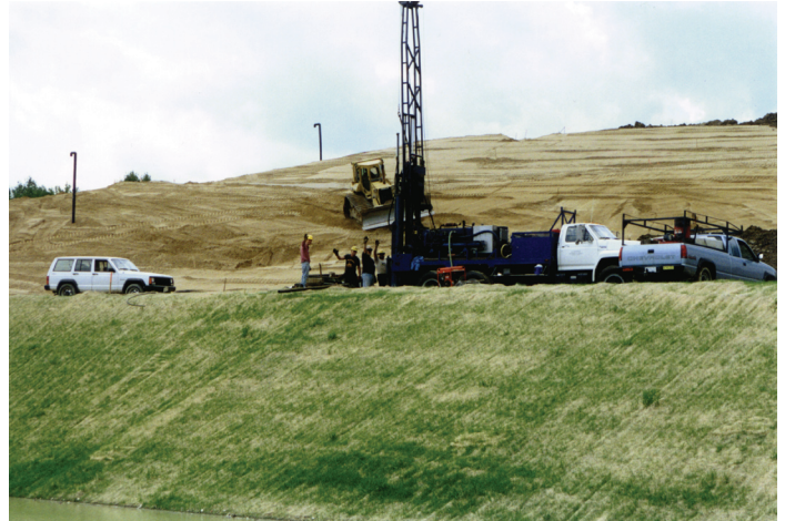
Photo 1. Drill rig installing monitor well at Saco Area 4 Landfill (landfill forms hill in background).
