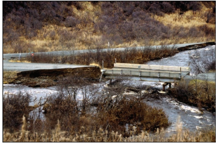
Road damage, Ninilchik River at Ninilchik, Alaska, October 25, 2002. Photograph taken by David F. Meyer, U.S. Geological Survey.
