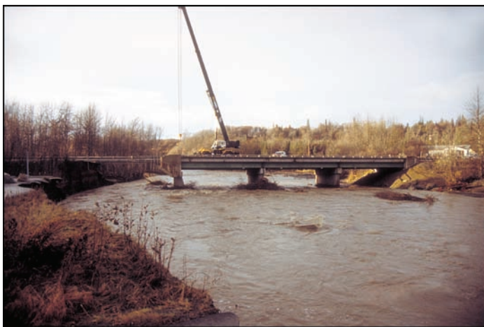
Bridge damage, Sterling Highway at Deep Creek near Ninilchik, Alaska, October 25, 2002. Photograph taken by David F. Meyer, U.S. Geological Survey.
