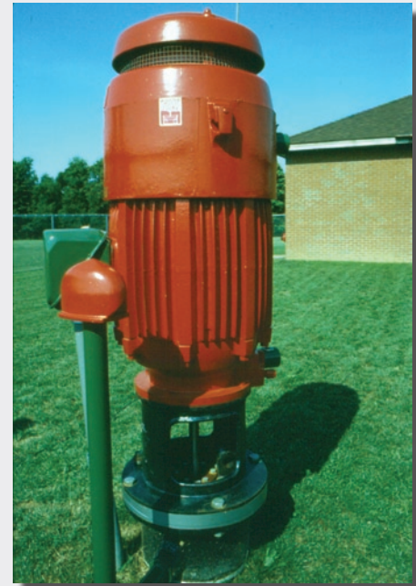
A supply well in Cortland aquifer
