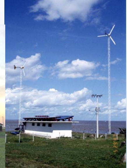
Brazilian hybrid power system
