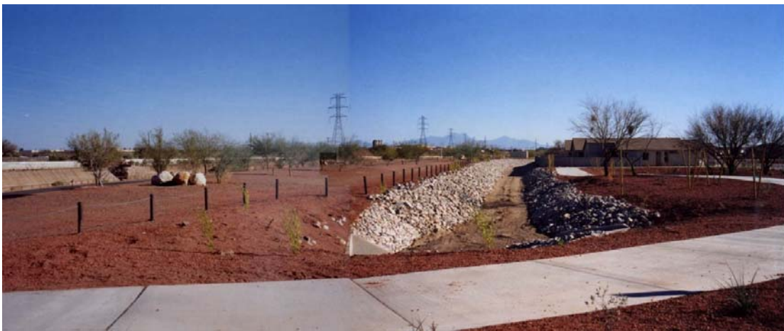
New housing and drainage structures on the Santa Cruz west bank south of Ajo Way
