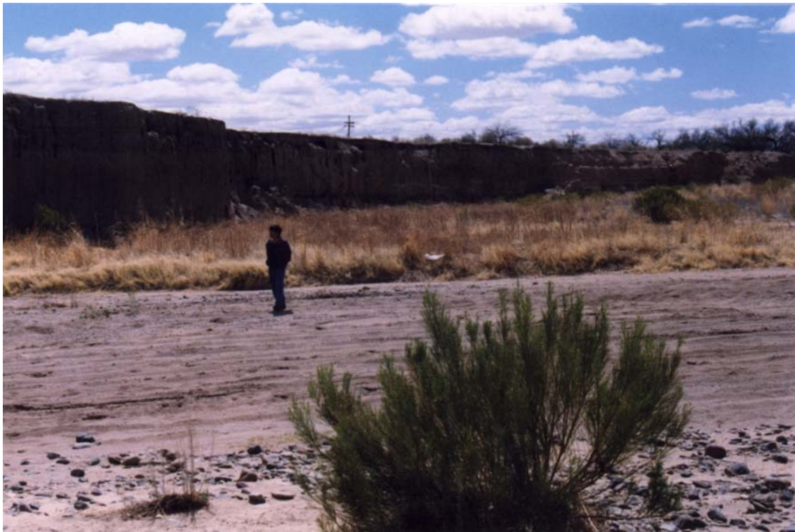
Note the nearly vertical banks in this unprotected reach south of Drexel
