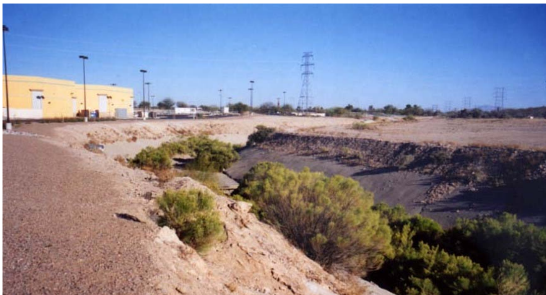
Condition of tributary wash upstream of its confluence with the Santa Cruz River
