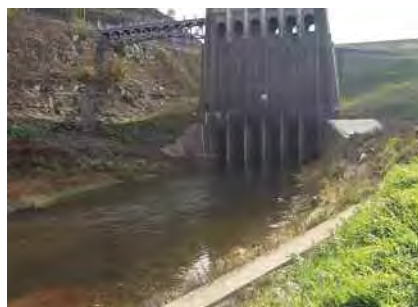
Mohawk Dam was authorized by the Flood Control Act of 1938 and was built along with 13 other dams to control flooding within the Muskingum River watershed. Work was done by the Civilian Conservation Corps, WPA, during the great depression. From: www.lrlh.usace.army.mil/_kd/go.cfm?destination=Page&Pge_ID=1227 .
