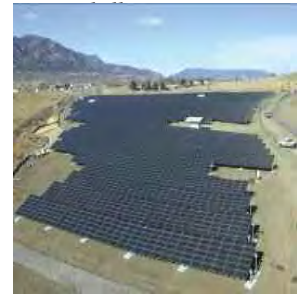
The largest solar power site in the Army, constructed on a closed landfill, will soon supply power to Fort Carson, Colo.
