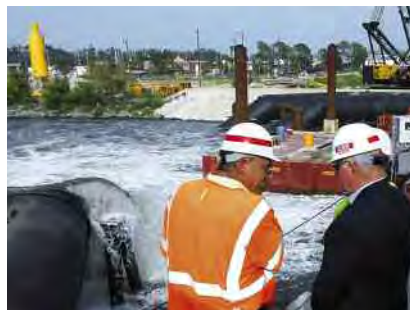
Former Secretary of the Army Dr. Francis J. Harvey is briefed by U.S. Army Corps of Engineers officials at the 17th Street Outfall Canal and Pumping Station in New Orleans Oct. 2, 2006. Harvey toured flood-ravaged New Orleans and USACE's efforts to repair the damaged facilities. Photo by: Betsy Weiner. Date: October 5, 2006. Courtesy of US Army from: http://www4.army.mil/OCPA/uploads/large/2006/OCPA-2006-10-05-131652.jpg .
