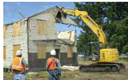
Workers remove a panel from a building at Fort Lewis, Wash., during modular deconstruction. Photo by Rebekah Barker. Date: Feb. 05, 2007. Photo courtesy of US Army from: http://www.army.mil/images/2007/02/05/2394/ .
