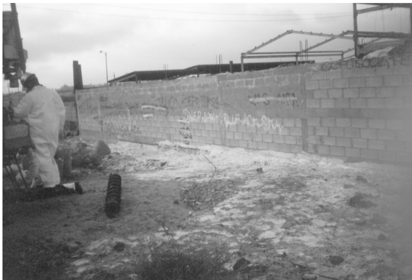
Photo No. 1: Outside view of waste pile containment wall south of plant
