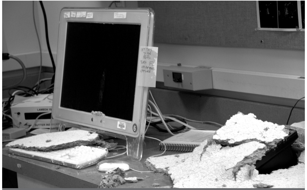
Wet ceiling tile debris fell on top of several computers and phones in workspaces on the B2 level.
