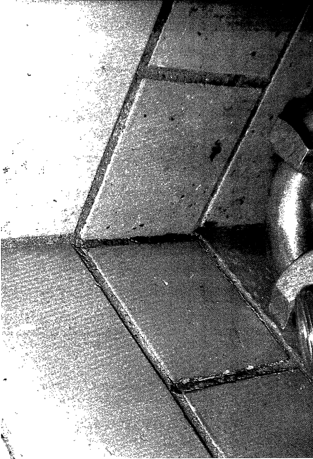
Cockroach-type insects creeping up the corner wall behind the pasteurizer and homogenizer in an ice-cream firm. Over 25 roach-type insects were noted in this area during the inspection.
