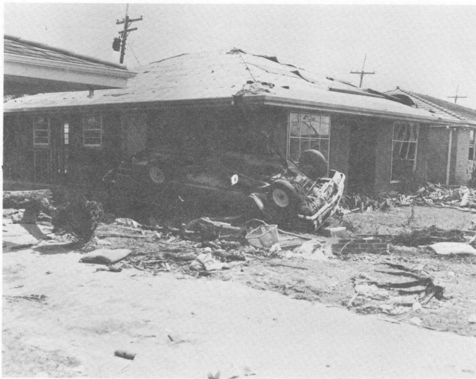
WATER AND WIND DAMAGE NEW ORLEANS, LA.
