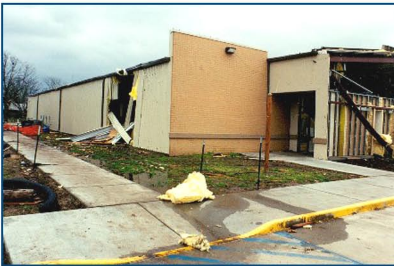
Severe damage to metal stud walls of the hospital's clinic building.
