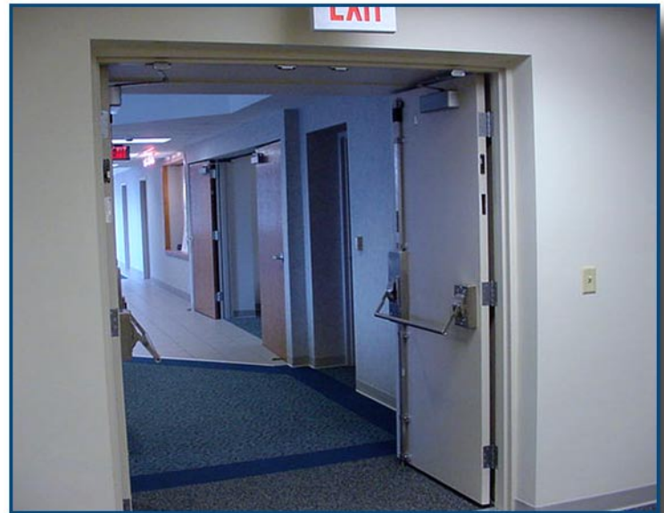
The double door without mullion allows hospital staff to move patients in rolling beds into the shelter.
