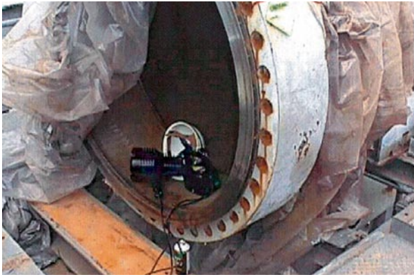
Figure 4-2. Pipe in which worker was asphyxiated
