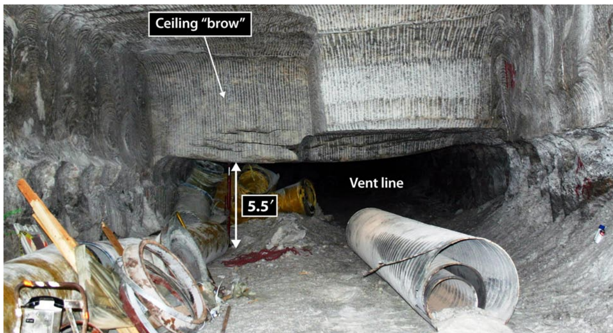
Figure 2-1. Vent pipe in the drift
