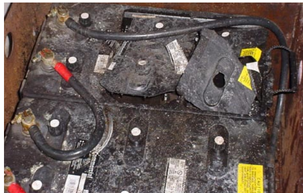
Figure 4-2. Damaged top of failed battery cell
