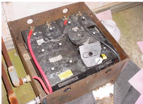
Figure 4-1. Battery box containing failed battery
