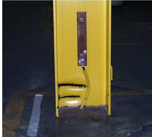
Figure 1-2. Penetration damage from forklift tines
