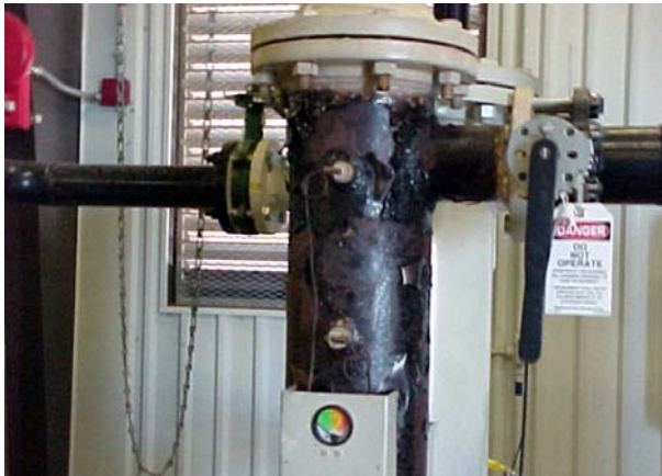
Figure 3-2. Fire-damaged filter housing
