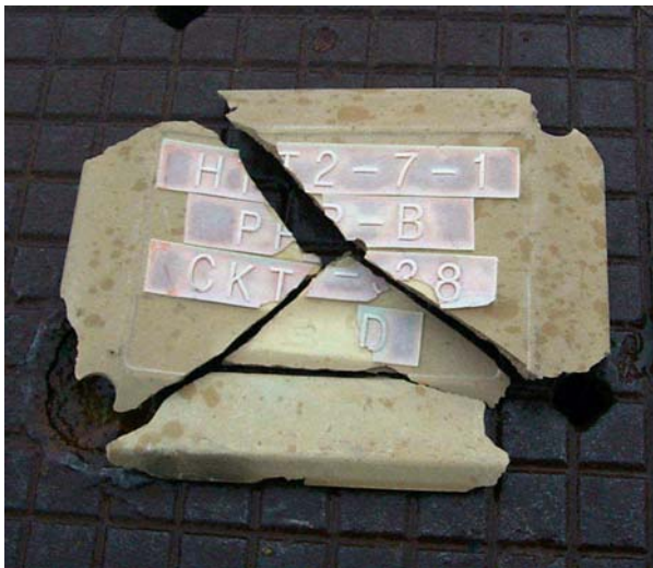
Figure 3-2. Shattered junction box cover
