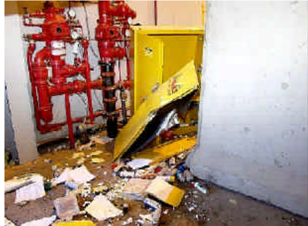
Figure 3-2. The damage to the flammable materials storage cabinet
