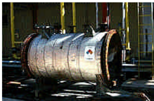
Figure 3-4. The opened process vessel
