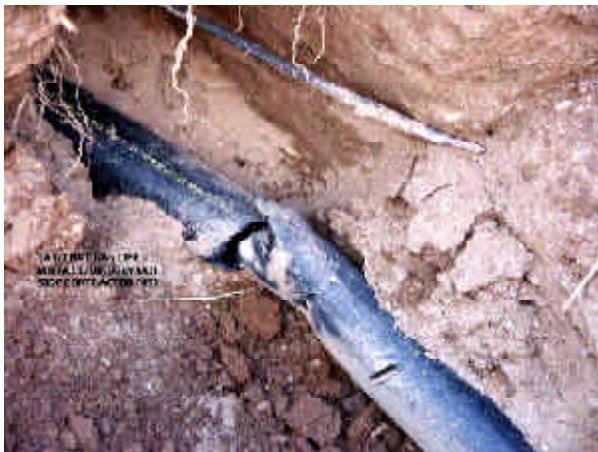
Figure 1-1. Cut gas line
