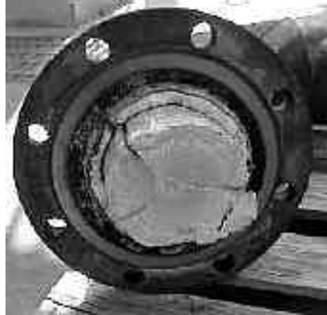
Figure 3-7. The vent pipes were plugged with hardened material
