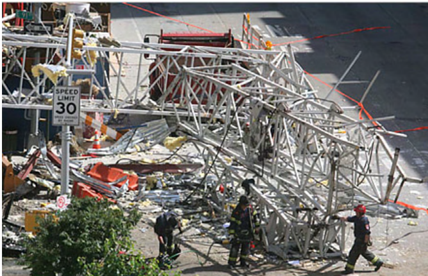
Figure 1-4. Crane on ground following May 30, 2008, accident
