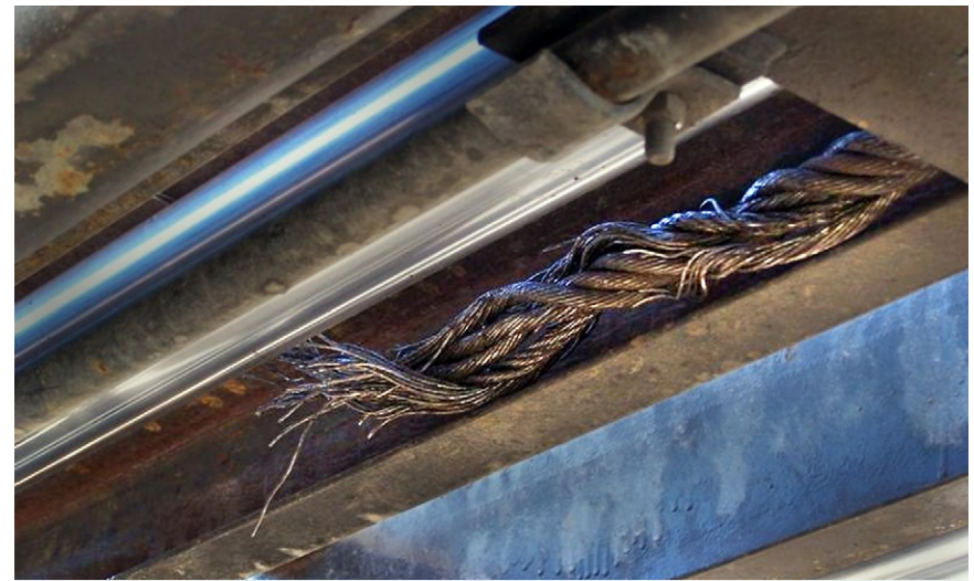
Figure 1-3. Broken cable underneath the truck rails
